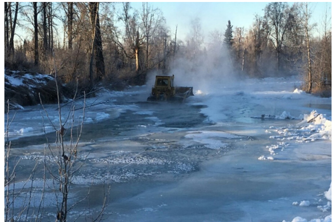
Fig. 5. Bulldozer deployed in the shallow Ship Creek affected by early-season ice formation near Anchorage, Alaska (Photo credit: Steven Daly, December 2016).
