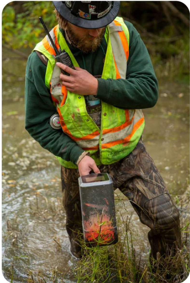
A ROHL employee confirming GPS location of conduit that's been installed by horizontal directional drilling.
