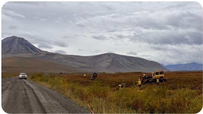
Installation of fibre optic conduit using a low-pressure vehicle called a Rolligon plow. This ensures that the delicate tundra habitat is minimally disturbed.
