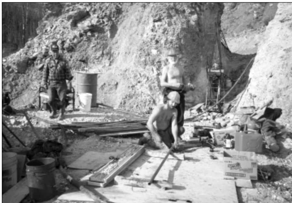
Figure 22. AX drilling rig at the Shootamook Creek property of Yukon Yellow Metal.
