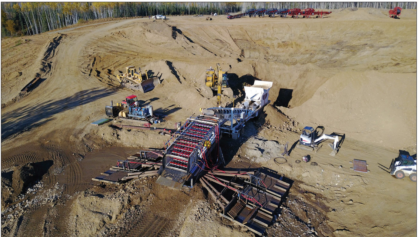
Figure 6. A view of the new wash plant and feeder being installed on Wolfhead Discovery and Mining's operation on lower Clear Creek.
