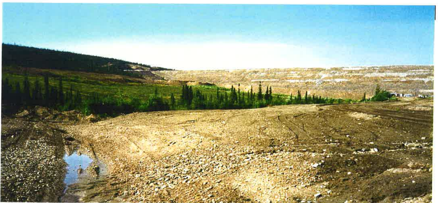
Figure 17: Looking up Fish Creek valley towards the tailing embankment, historically disturbed areas being recontoured during construction of Channel 1, Summer 1997
