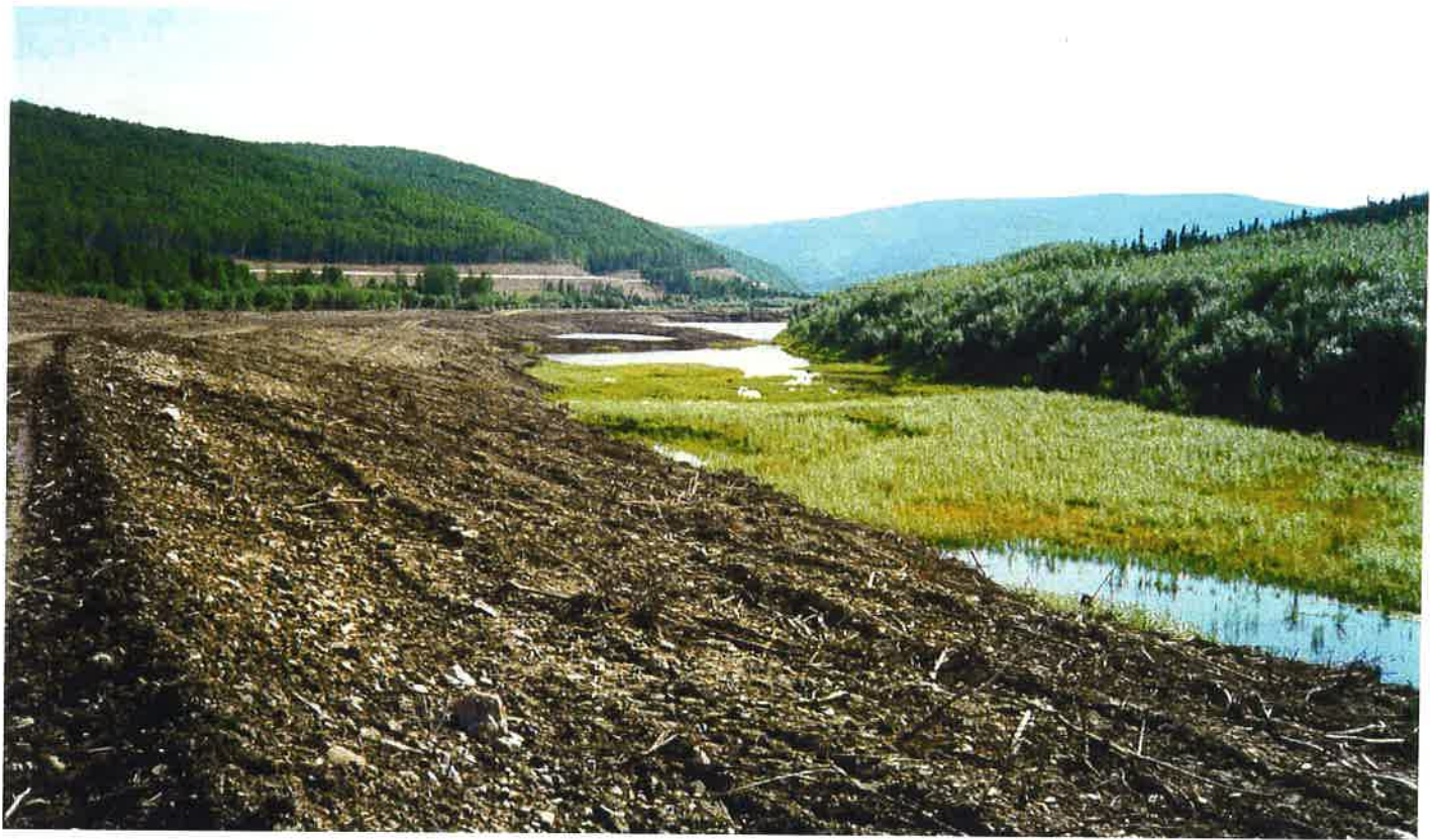
Figure 20: Steep sided pits and uneven terrain were sloped in preparation for seeding reclaimed wetlands downstream from the tailing impound, 1999
