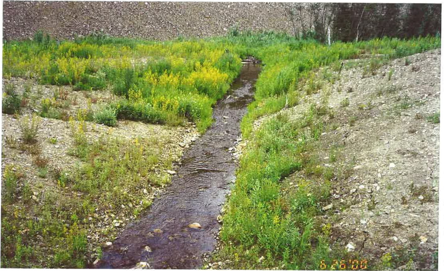
Figure 16: The shallow channel constructed to allow grayling to enter the wetlands for spawning, June 2000
