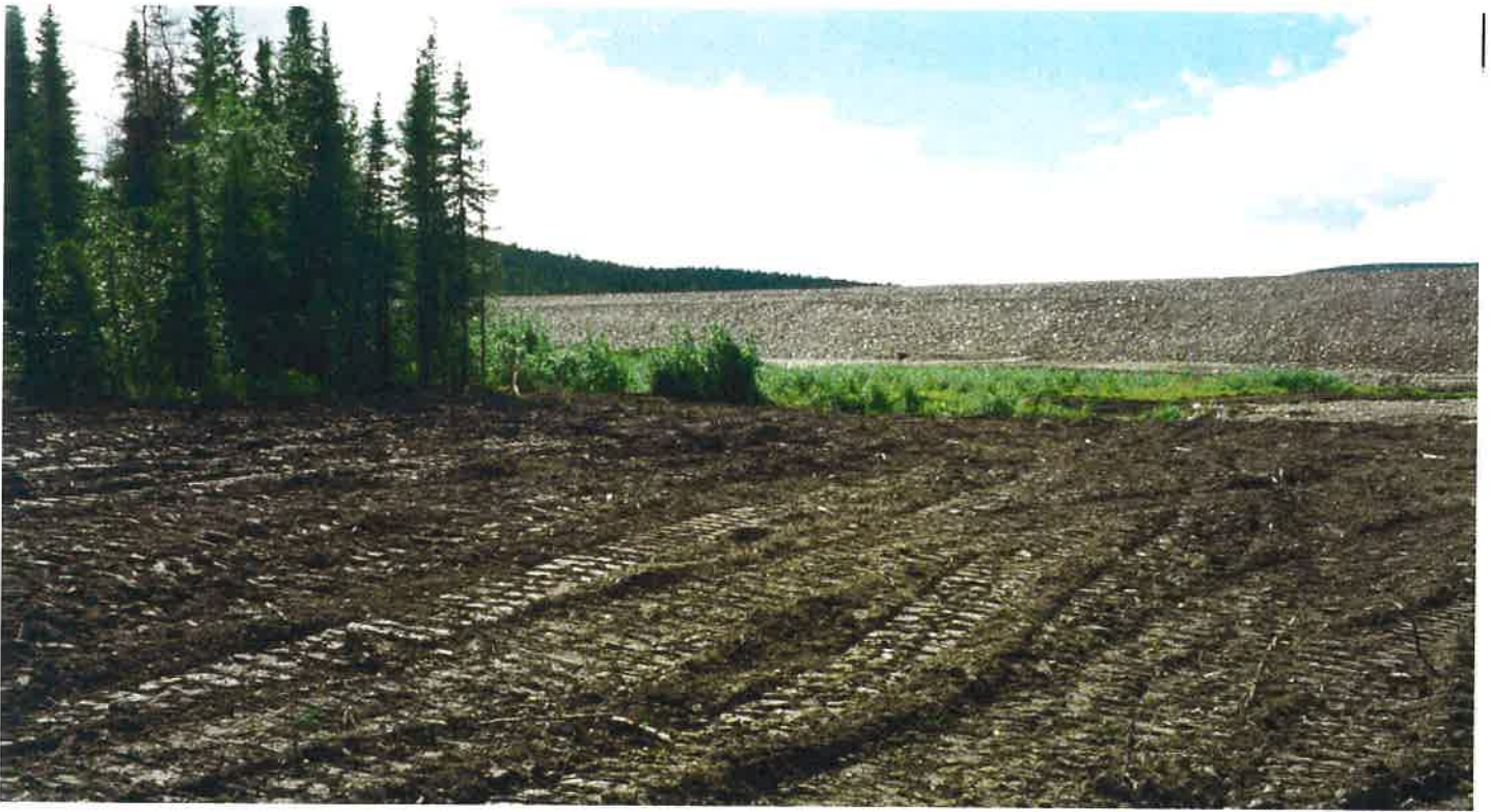
Figure 10: Below the water supply reservoir the area was recontoured and seeded after construction of the embankment, Summer 1996
