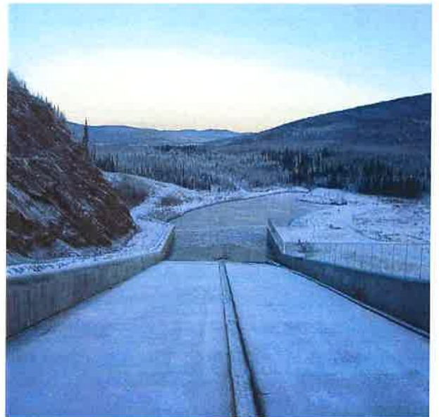
Figure 51: Water supply reservoir spillway/otter slide, in the bottom left corner of photo are faint slide marks left by playful otters, December 2002
