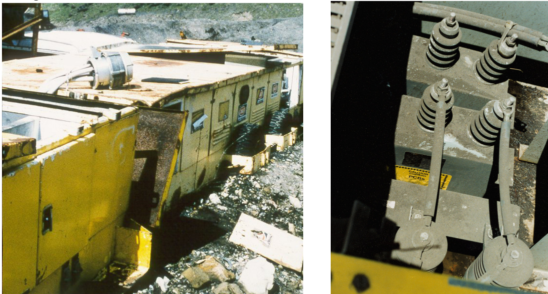
Fig. 6 Coal mine power center containing PCB capacitors
