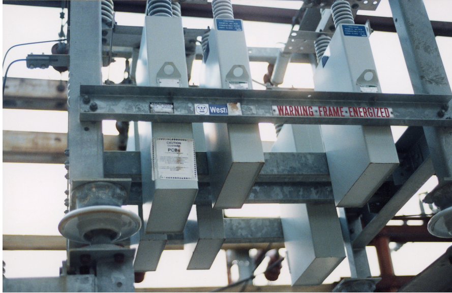
Fig. 3 PCB marked capacitor on the left
