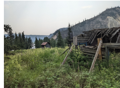
Rampart House, 2022. View to the SW from Paul George House at left, looking toward frame cache. Wendy Shearer photo
