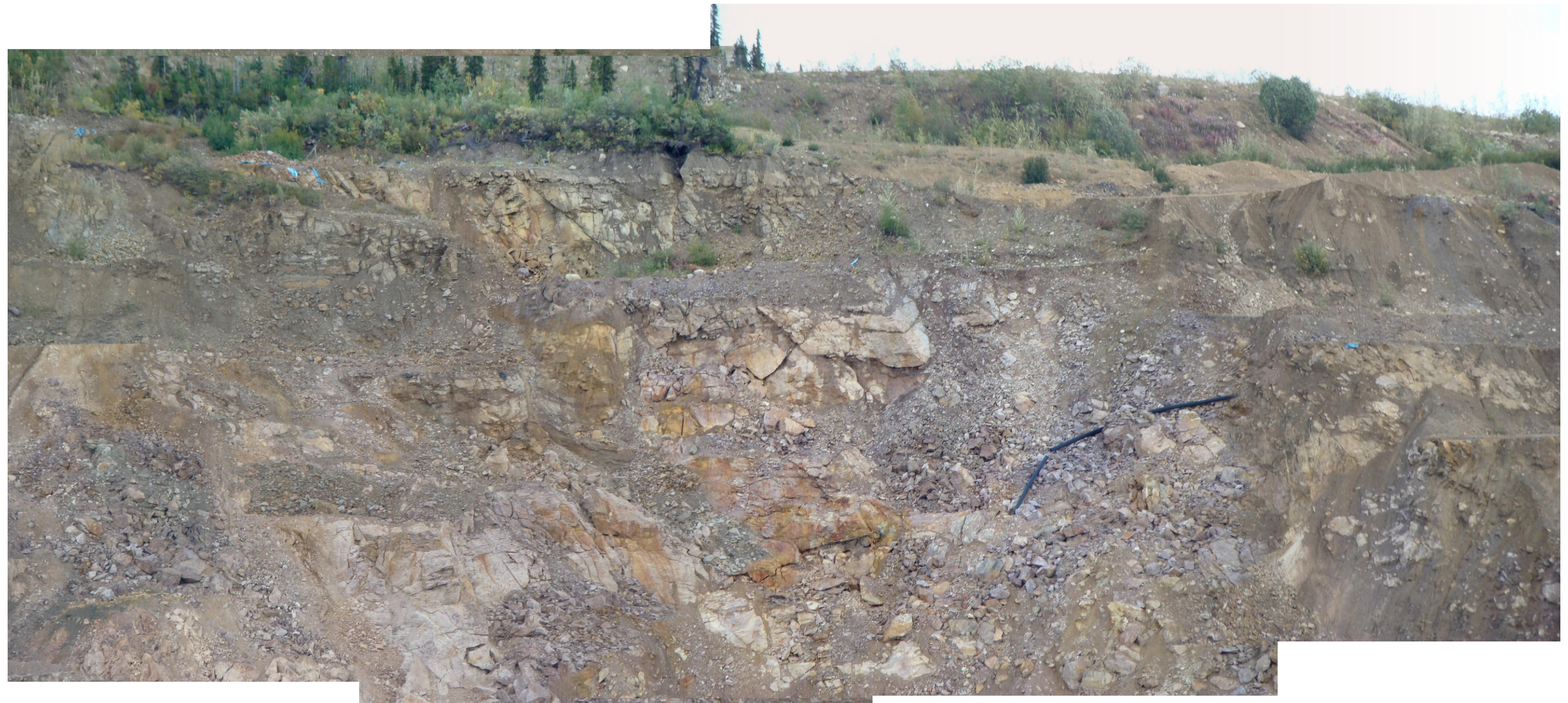
Photograph 13 : South instability zone. View of the crest of the pit wall. (August 2009).
