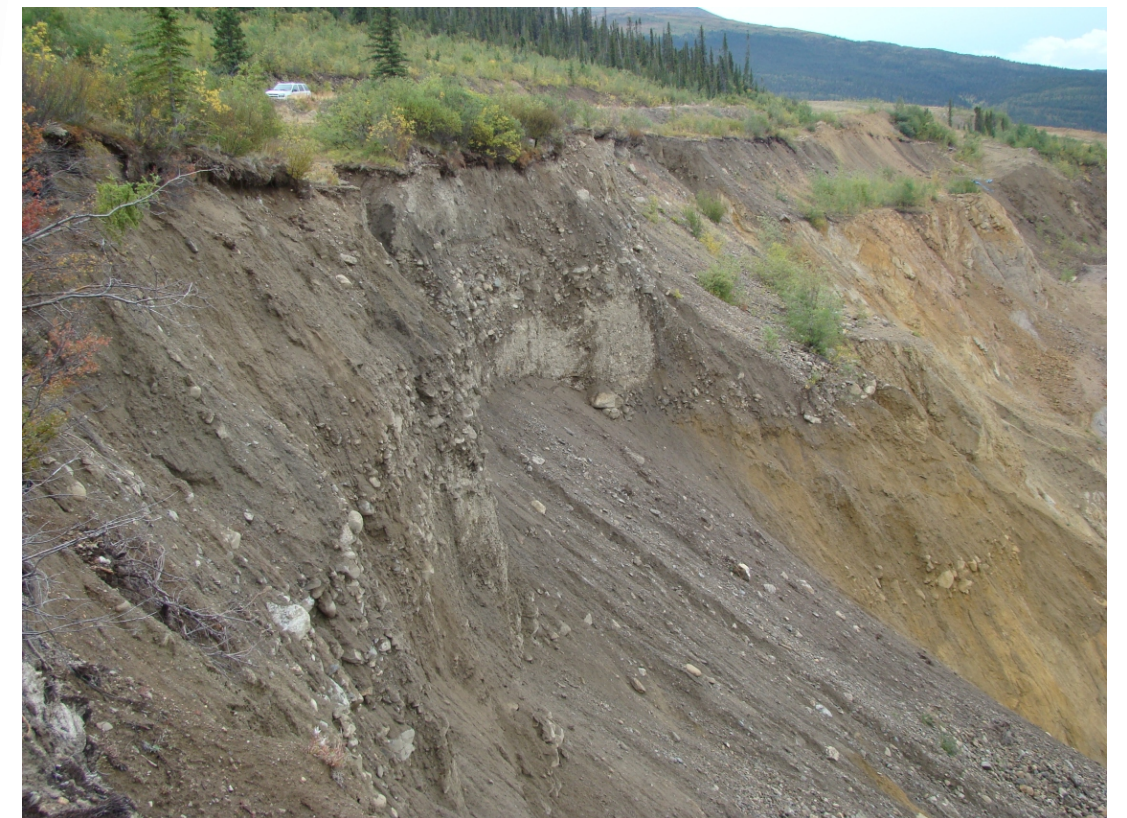
Photograph 8 : North instability zone. View of crest of the pit wall on overburden soils near reference bar 15355 (August 2009).
