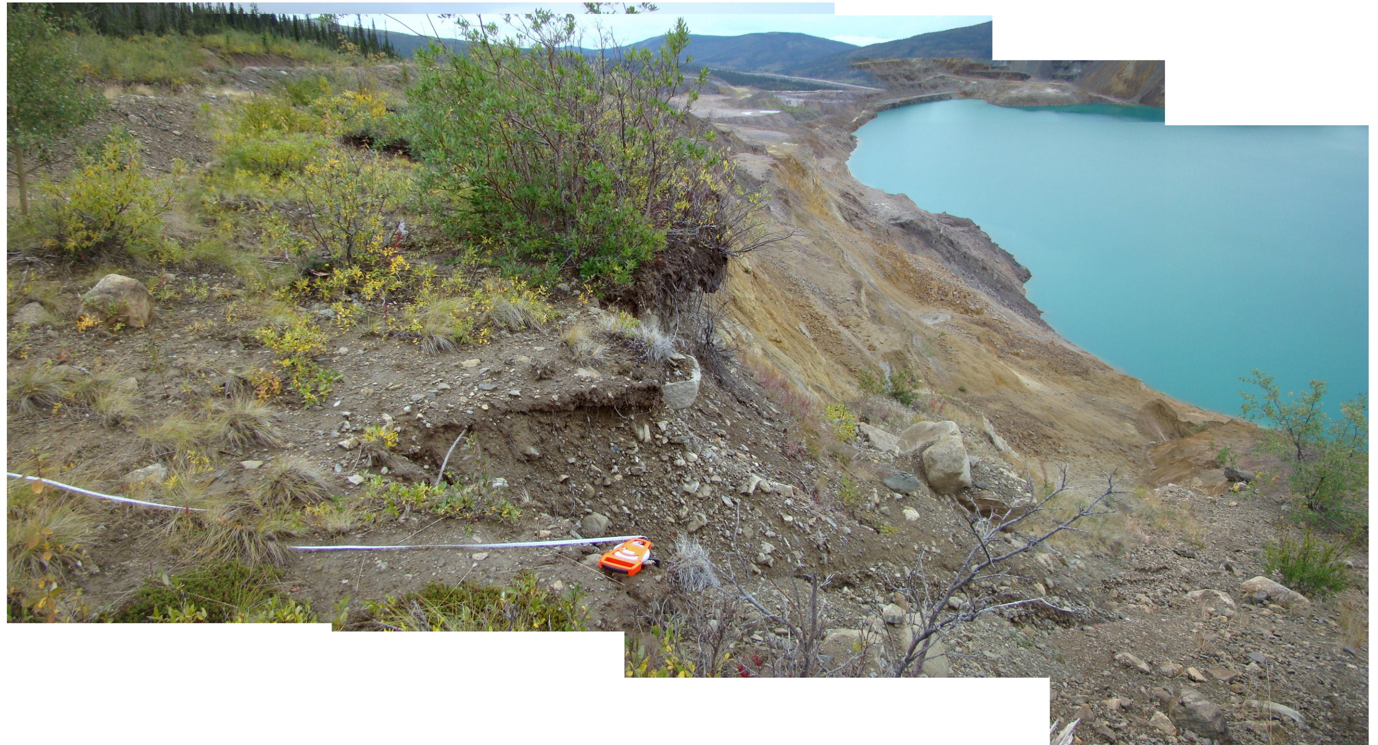
Photograph 6 : North instability zone. View of crest of the pit wall near reference bar 15354 (August 2009).
