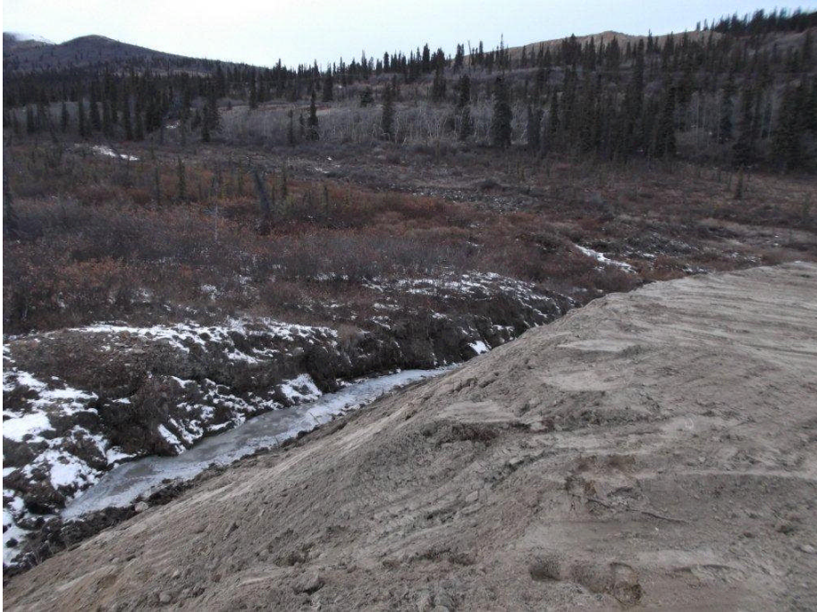
Photo 2: Flattened slope near Dome Creek (YG Photo, October 2012)
