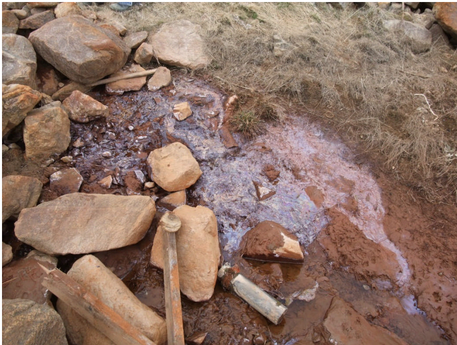
Photo 6: View of seepage from toe of tailings dam, just above the seepage collection pond (June 1/12)
