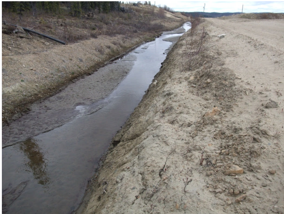
Photo 3: Low flow in diversion ditch due to silt and sand deposits (June 1/12)
