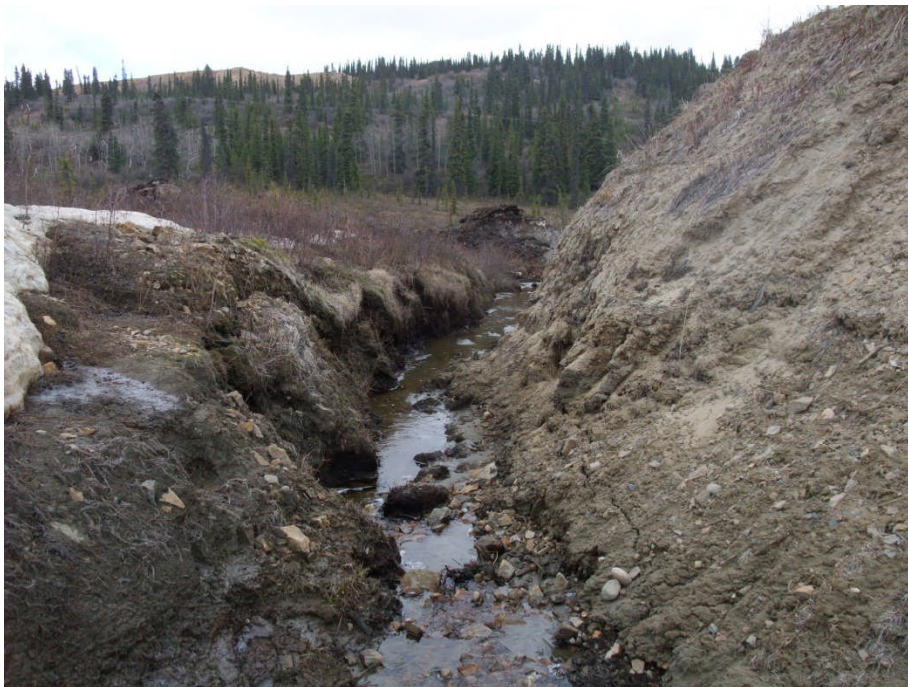
Photo 1: Oversteep ditch slope near Dome Creek (June 1/12)
