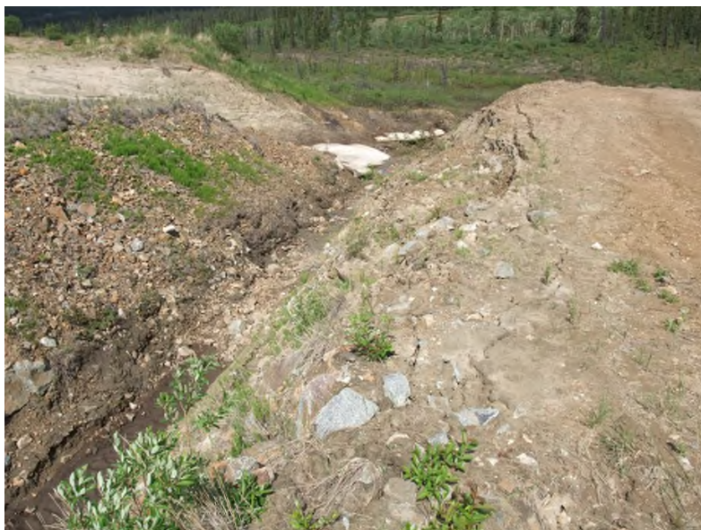
Photo 2: Oversteep ditch slope upstream of Dome Creek intersection (June 21/13)
