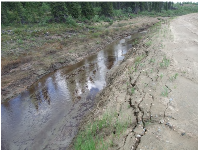
Photo 1: Oversteep ditch slope on Dome Creek Diversion (June 21/13)
