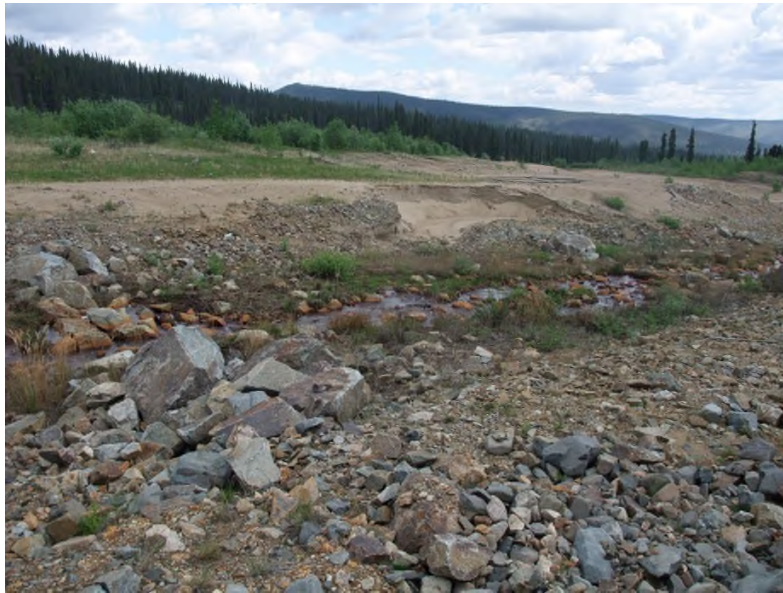
Photo 4: View of Erosion Scour on north side of spillway that must be repaired (June 21/13)
