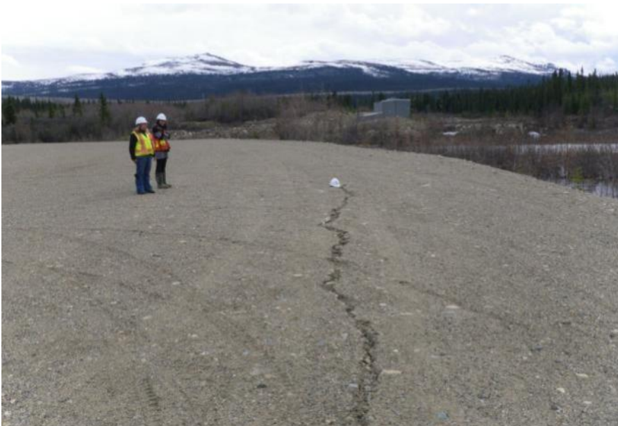
Photo 26 Longitudinal crack along downstream berm road surface towards Canal Dyke (May 29, 2012)
