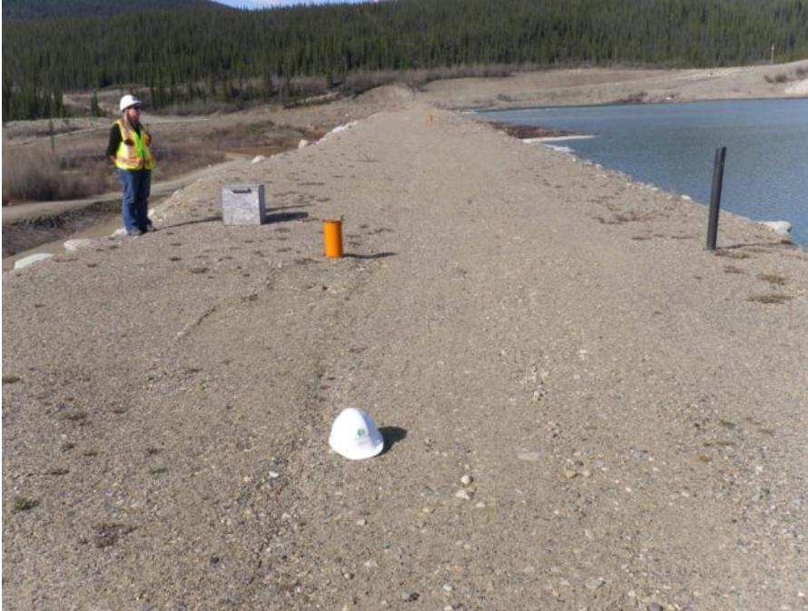
Photo 39 Longitudinal crack in the middle of crest along southwest segment (May 29, 2012)
