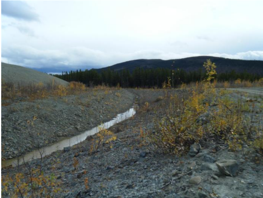
Photo 61 Vangorda Waste Dump Seepage Collection Ditch between Drains No. 3. and No. 4. (September 20, 2011)
