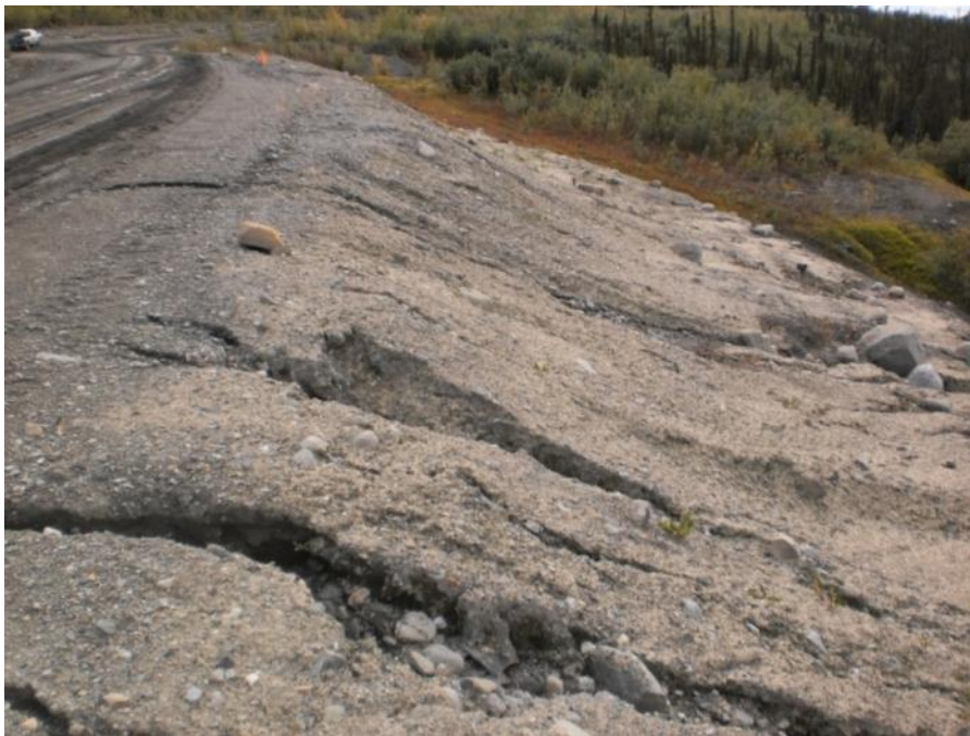
Photo 92 Gully erosions on downstream slope
