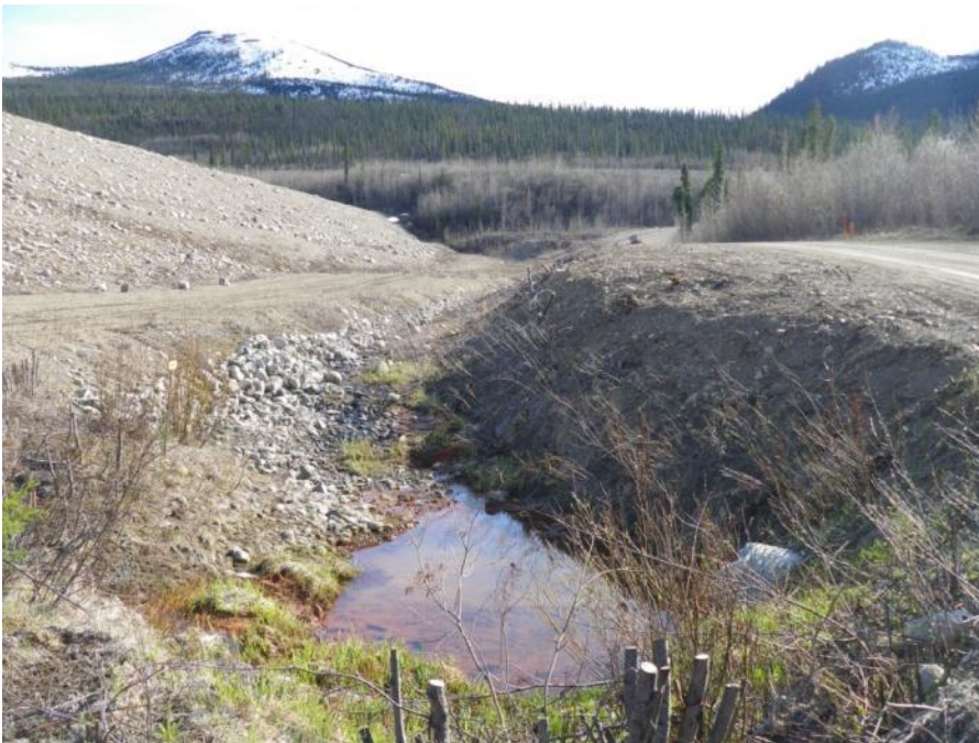
Photo 42 Downstream seepage along middle segment of dam (May 29, 2012)
