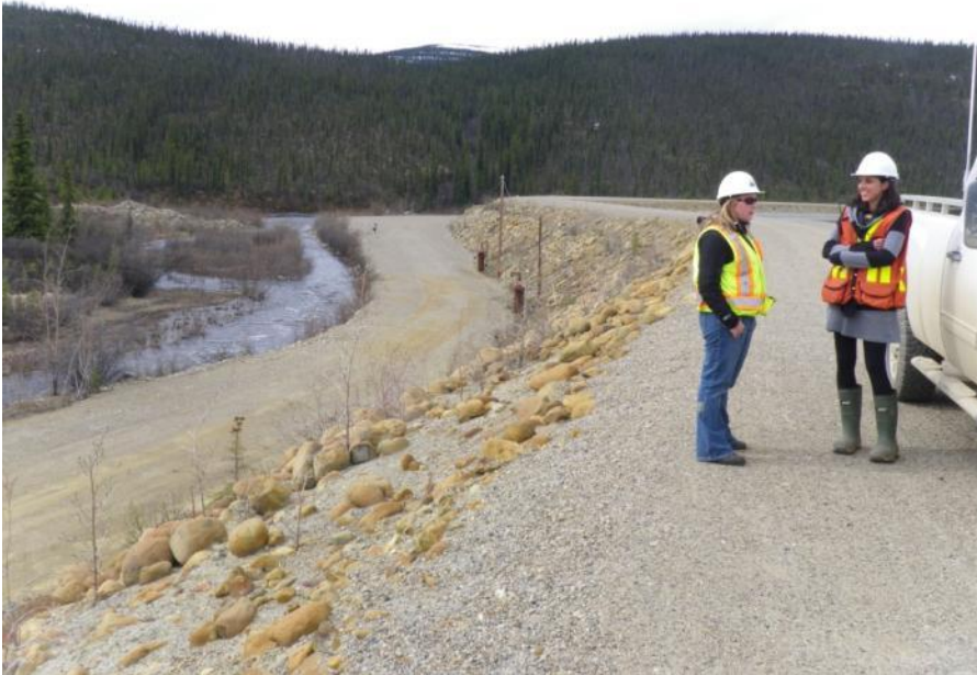
Photo 25 Secondary Tailings Dam crest and downstream slope - longitudinal cracks reappeared along road surface of downstream berm (May 29, 2012)
