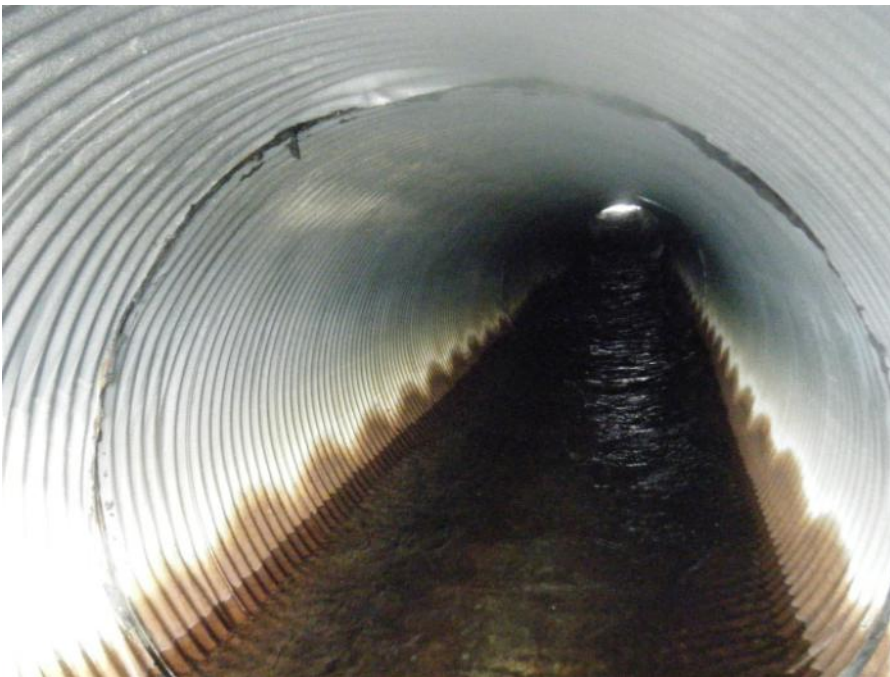
Photo 80 Vangorda Flume intake culvert as seen from downstream end - first pipe joint appears to be separated (September 20, 2011)
