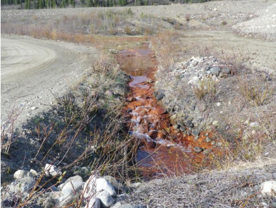
Photo 41 Downstream seepage along northeast segment of dam (May 29, 2012)
