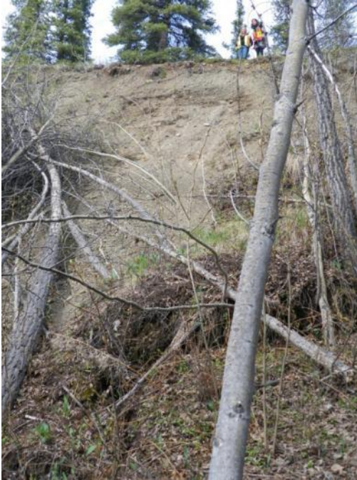
Photo 97 Downstream slope of esker - note seepage daylighting from slope (May 29, 2012)
