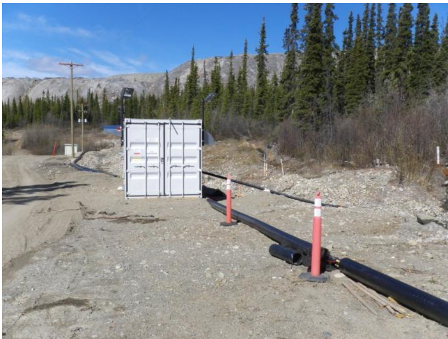
Photo 94 V-15 Enclosed Sump Pump for pumping excess water during spring freshet into Vangorda Pit (May 30, 2012)
