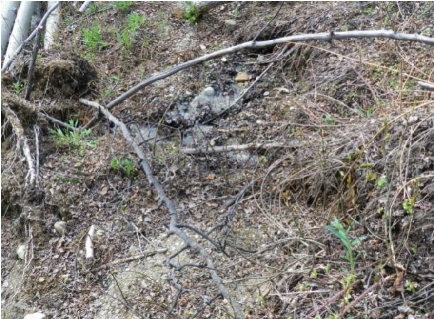
Photo 98 Seepage rate increased further down slope from the upslope daylighting location (May 29, 2012)
