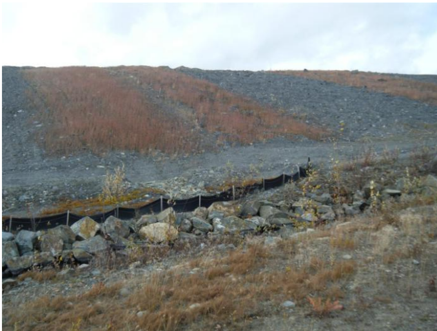
Photo 70 Grum Overburden Dump with vegetation test plots on dump face - Grum Interceptor Ditch in foreground (September 201, 2011)
