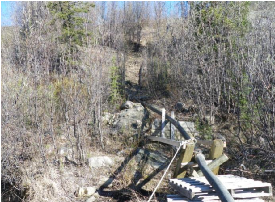
Photo 72 Pipeline below access road to convey collected surface runoff as seen on Photo 73 (May 30, 2012)
