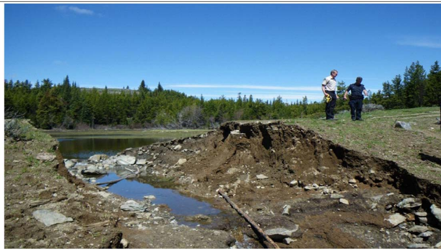
Figure 5 – Testalinden Dam Failure (near Oliver) June 13, 2010
