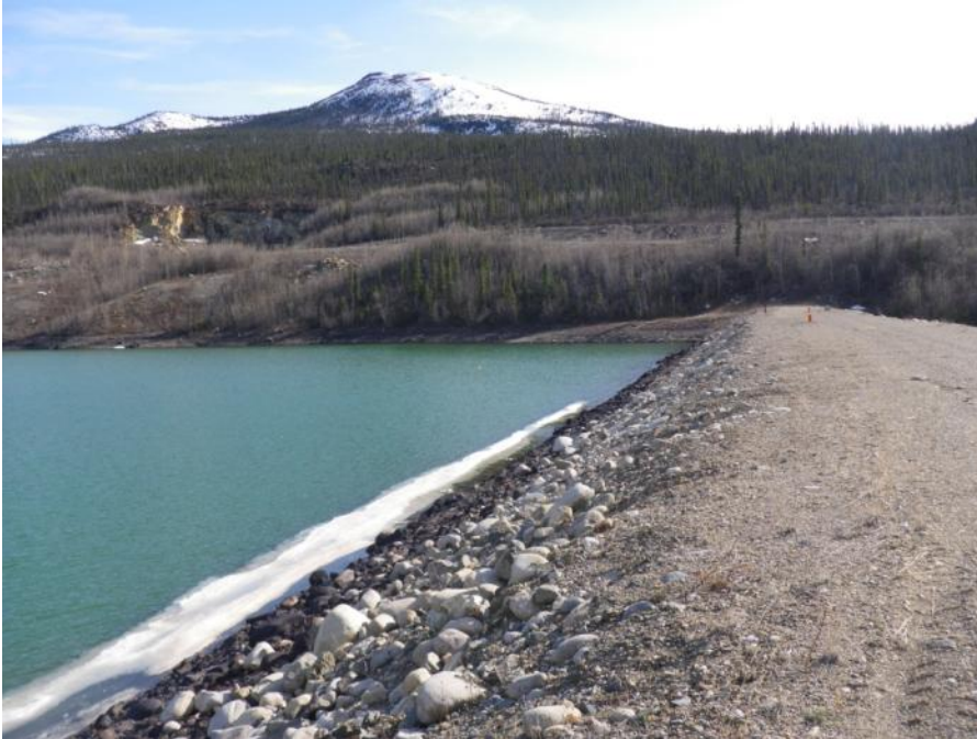
Photo 37 Cross Valley Dam crest and upstream slope (May 29, 2012)
