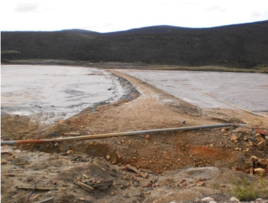
Photo 26 North end of Secondary Dam - a ditch in the foreground separating the dam with north abutment (August 23, 2011)
