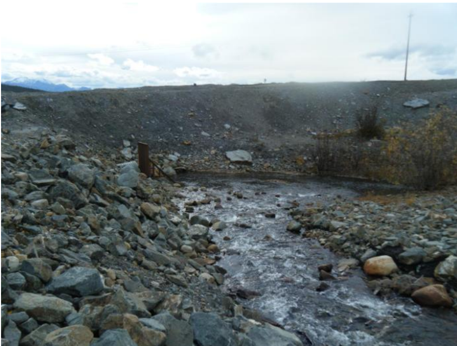
Photo 84 Vangorda Flume Plunge Pool and culvert to Vangorda Creek Diversion drop box (September 20, 2011)
