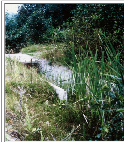
Figure 13 – Obstructed spillway channel
