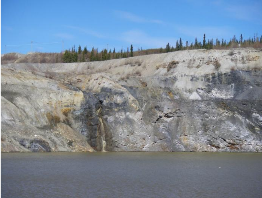
Photo 47 Vangorda Pit northwest wall lower segment - note Vangorda Flume behind the wall (May 30, 2012).
