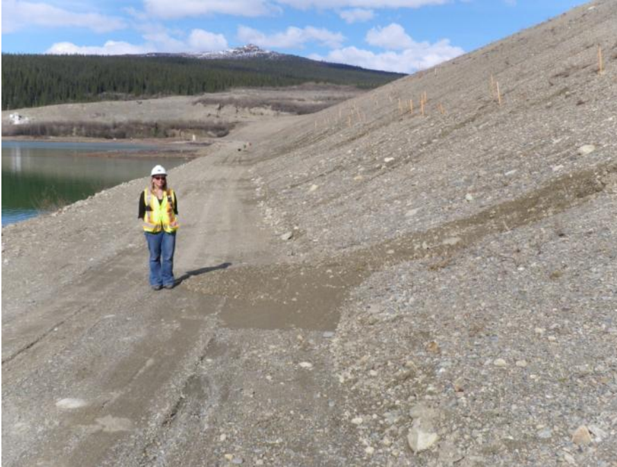
Photo 33 Rill erosions along downstream slope - note stakes used to assist ongoing monitoring by DES and deposits of eroded damfill on downstream berm surface (May 29, 2012)
