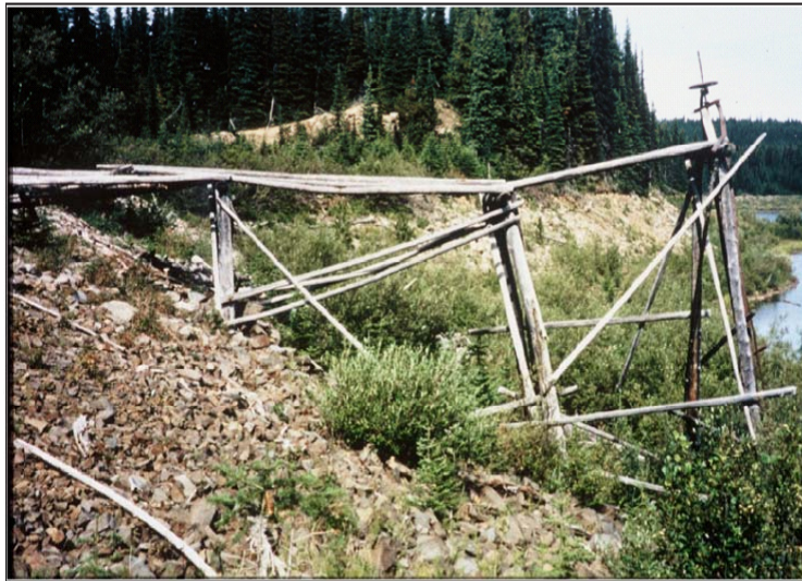
Figure 19 – Intake Control Access Structure Failure
