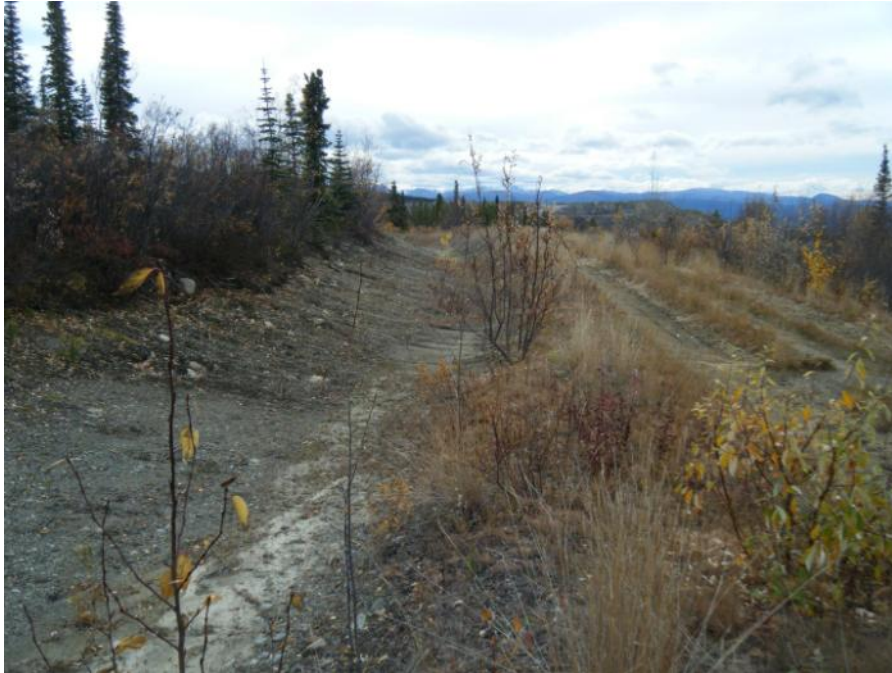
Photo 71 North-East Interceptor Ditch near its upstream end. Excavator bucket marks indicate recent cleaning of the ditch (September 20, 2011)
