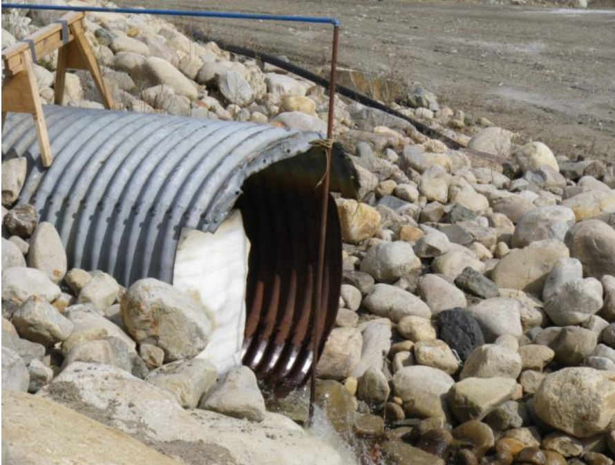
Photo 15 Discharge end of culvert leading to lower reach of Interceptor Ditch - note snow remaining inside culvert (May 30, 2012)
