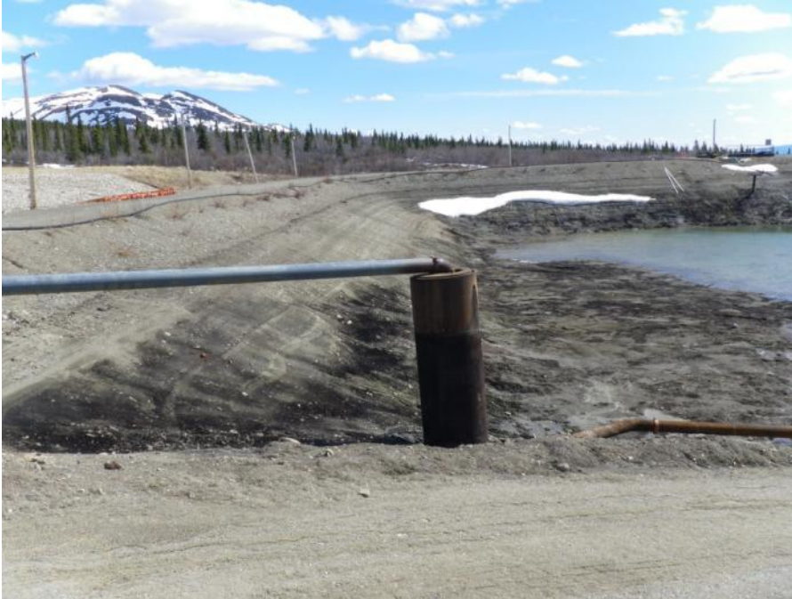
Photo 101 Sludge Pond and sludge inflow pipe - note freshly removed sludge surface (May 30, 2012)
