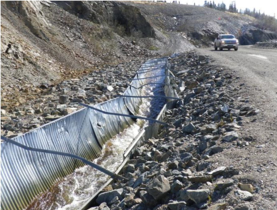
Photo 75 Battered section along lower reach of Vangorda Flume (May 30, 2012)
