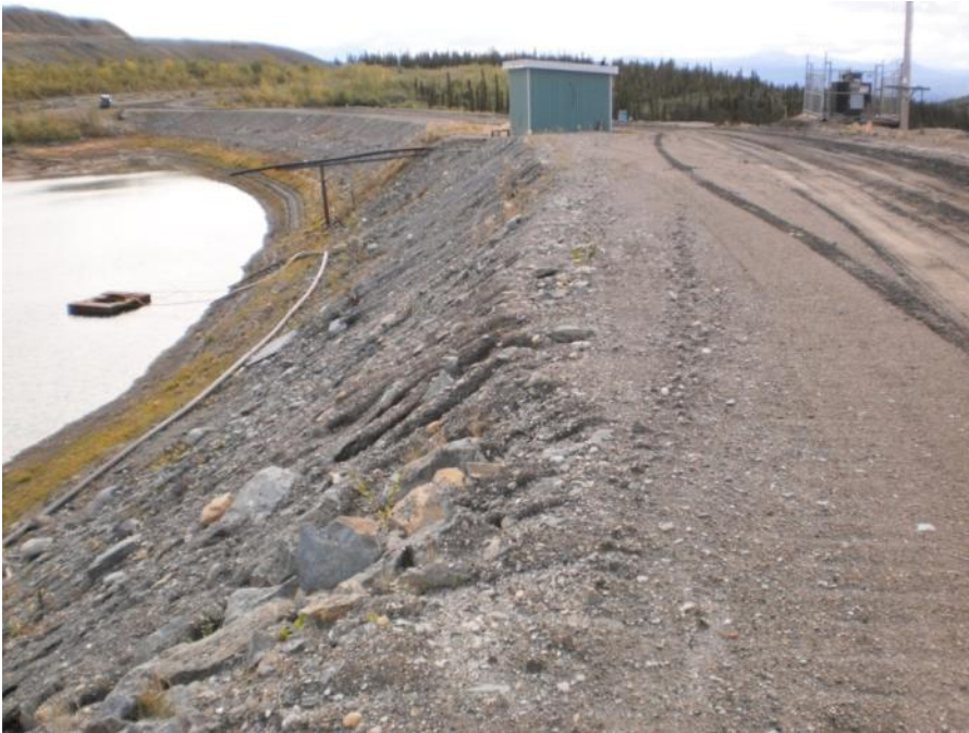
Photo 93 Dam crest and upstream slope - rill erosions in the foreground (August 23, 2011)
