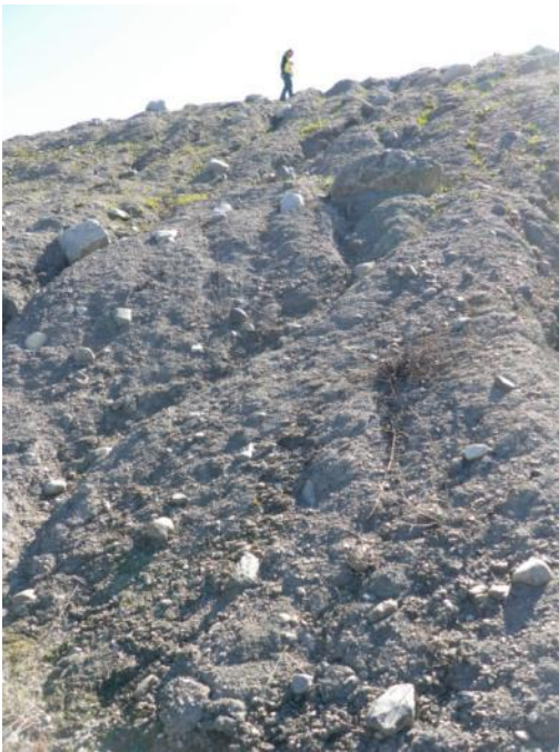
Photo 84 Downstream slope rill erosions (May 30, 2012)
