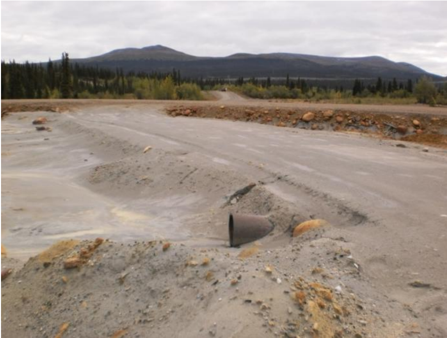
Photo 21 Junction of Original Tailings Dam (foreground) and Secondary Tailings Dam (background, August 23, 2011)
