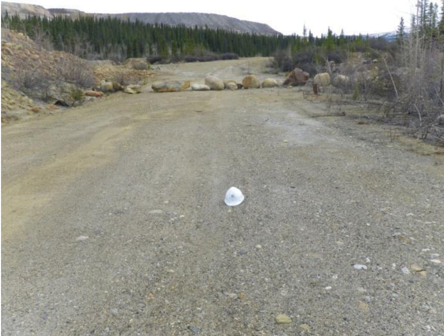
Photo 27 Longitudinal crack along downstream berm road surface towards Mine Access Road (May 29, 2012)
