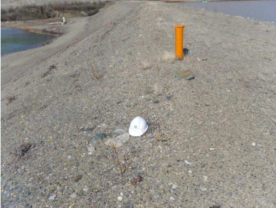
Photo 35 Sign of damfill adjustment near area of hard hat along crest shoulder (May 29, 2012)
