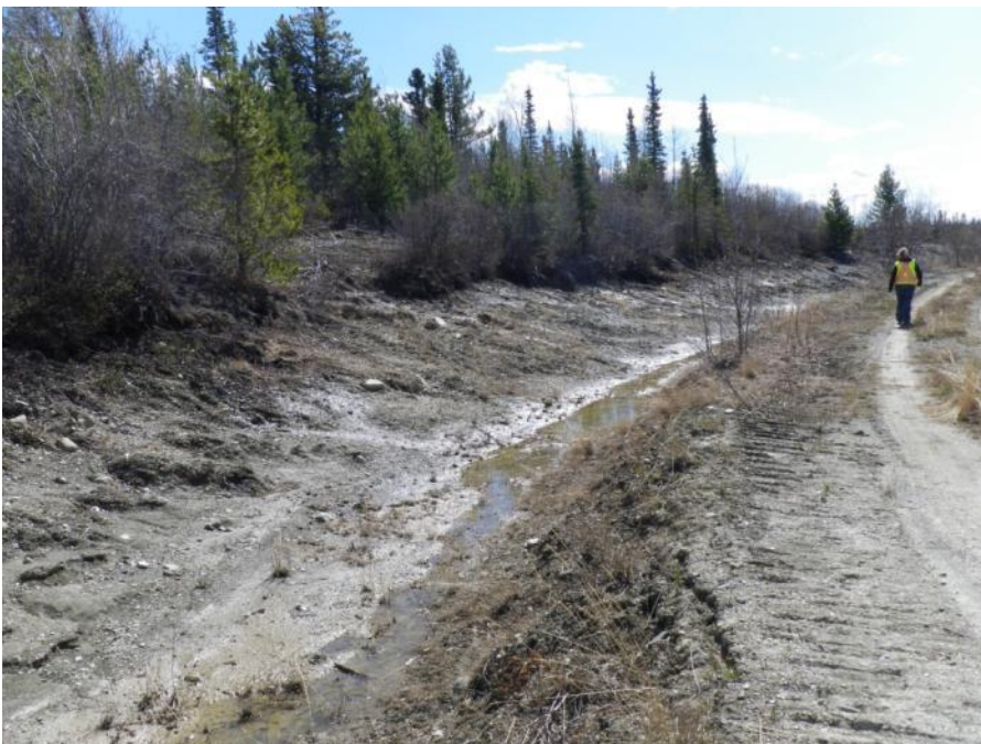
Photo 64 Ditch bank slopes – note bank slope erosion condition (May 30, 2012)
