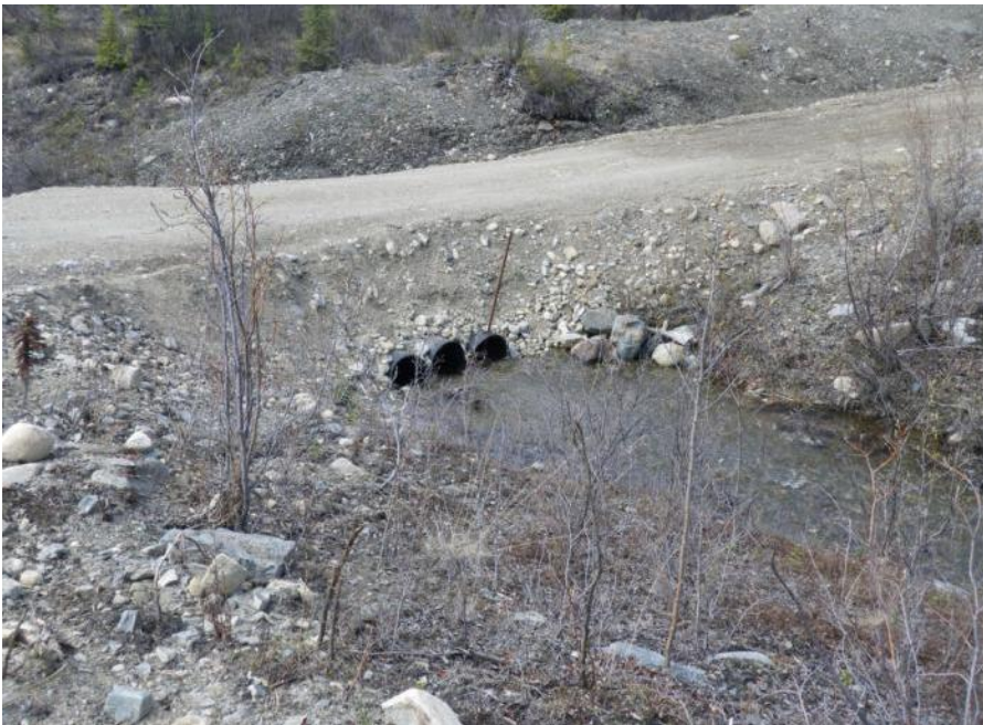
Photo 8 Channel upstream of Potable Water Well access road culverts - note sediment deposits at channel bottom (May 30, 2012)
