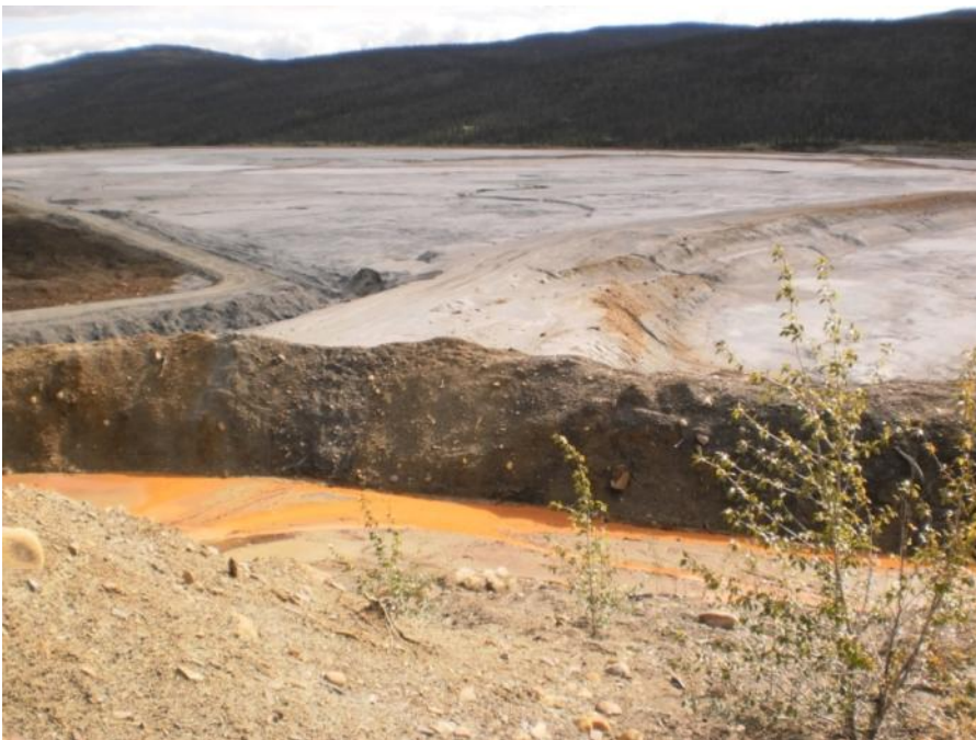
Photo 22 North end of Original Tailings Dam - a ditch in the foreground separating the dam with north abutment (August 23, 2011)
