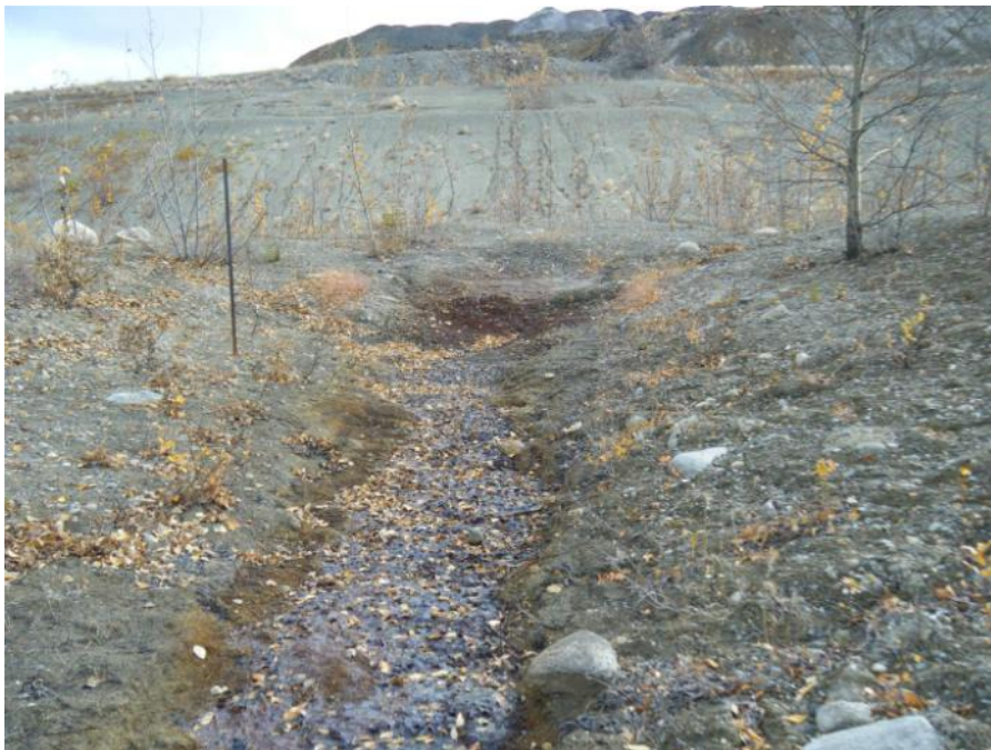
Photo 62 Vangorda Waste Dump Drain No. 4 - no weir at this drain (September 20, 2011)
