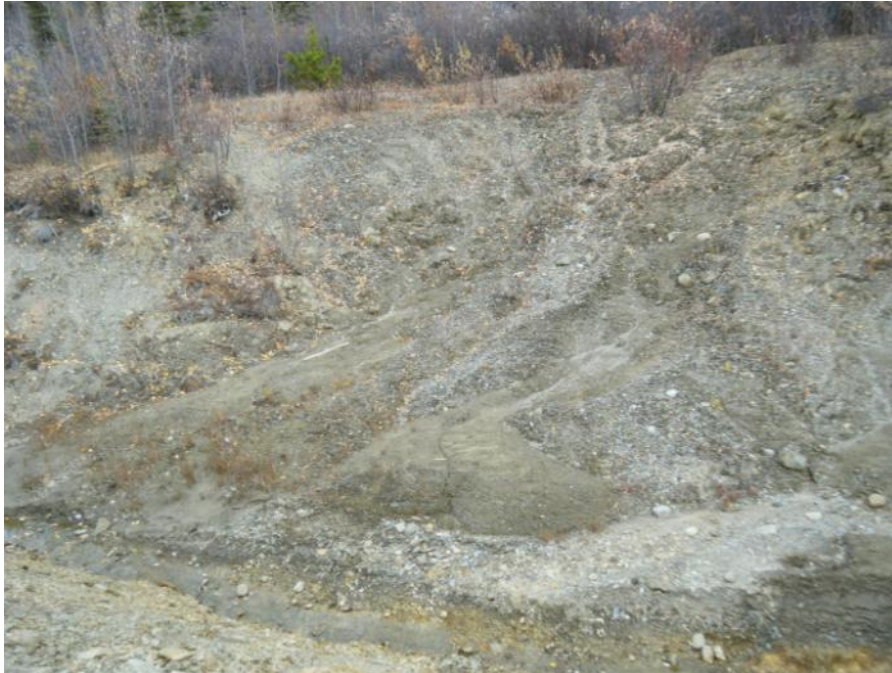
Photo 73 North-East Interceptor Ditch - note slumped side slope (September 20, 2011)
