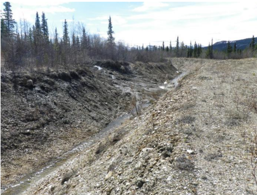
Photo 66 Ditch bank slope slump (May 30, 2012)
