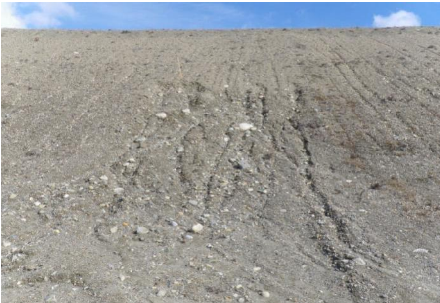
Photo 34 Rill erosions along downstream dam slope (May 29, 2012).
