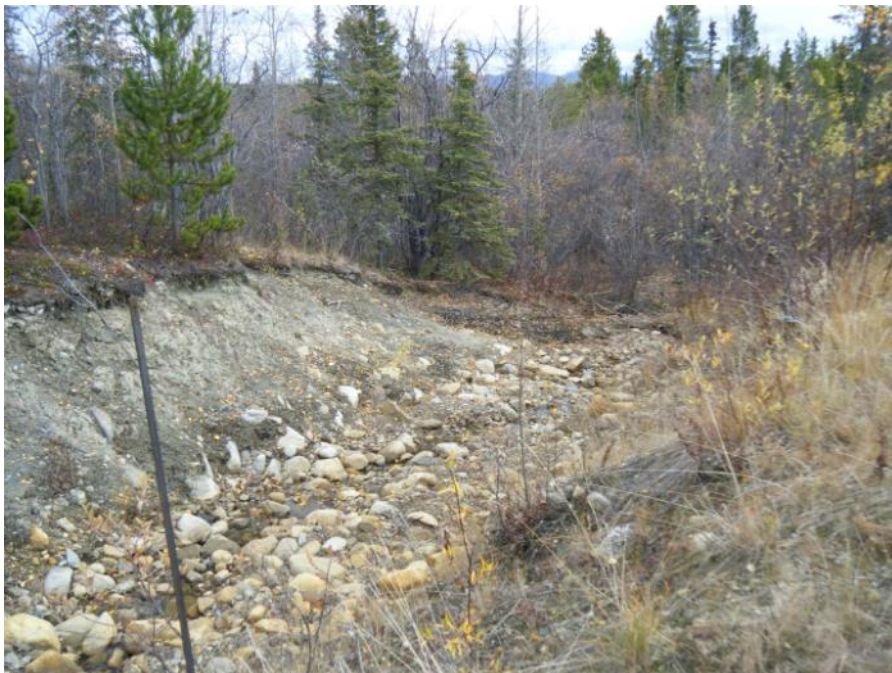
Photo 74 North-East Interceptor Ditch at its downstream end (September 20, 2011)
