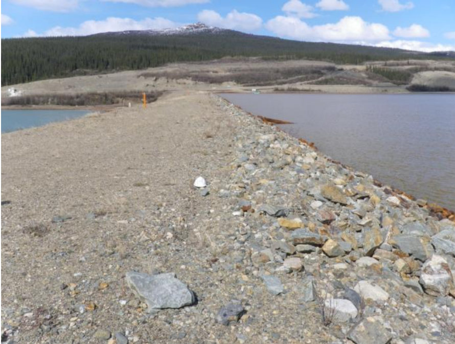
Photo 31 Dam crest and upstream slope - note damfill adjustment in area of hard hat along upstream crest shoulder (May 29, 2012)
