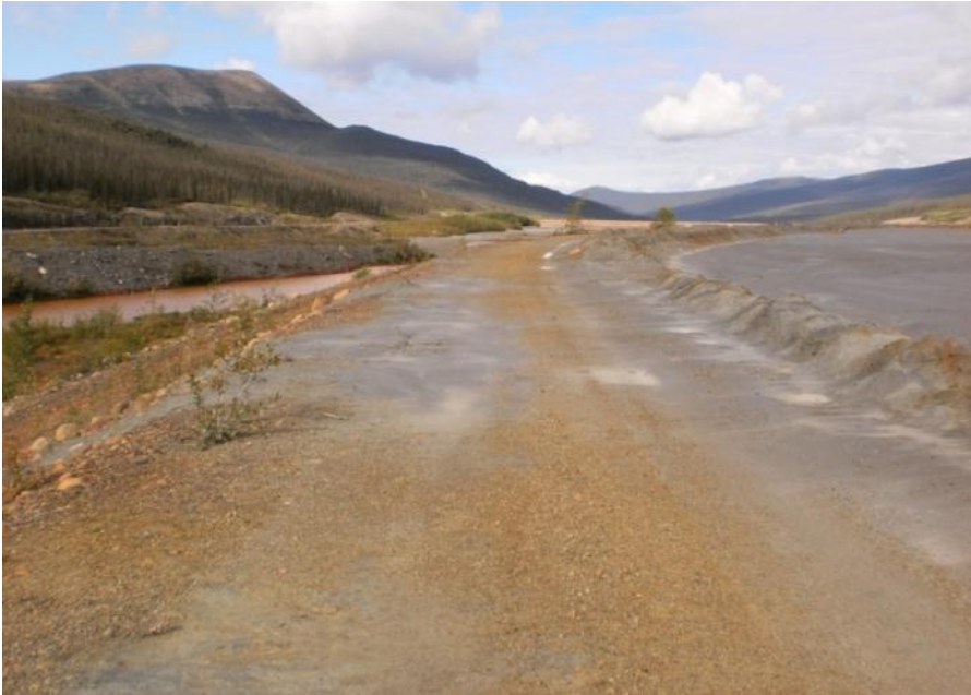
Photo 25 Dam crest near the vicinity where the diversion channel and tailings dam alignment begin to diverge – note tailings pile along upstream crest shoulder (August 23, 2011)
