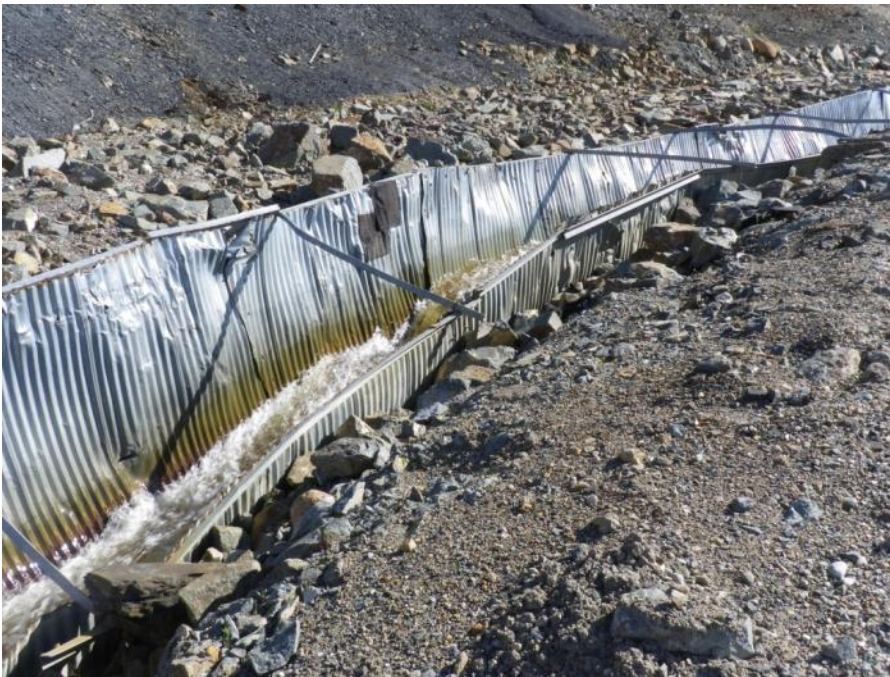
Photo 76 Battered section along lower reach of Vangorda Flume (May 30, 2012)
