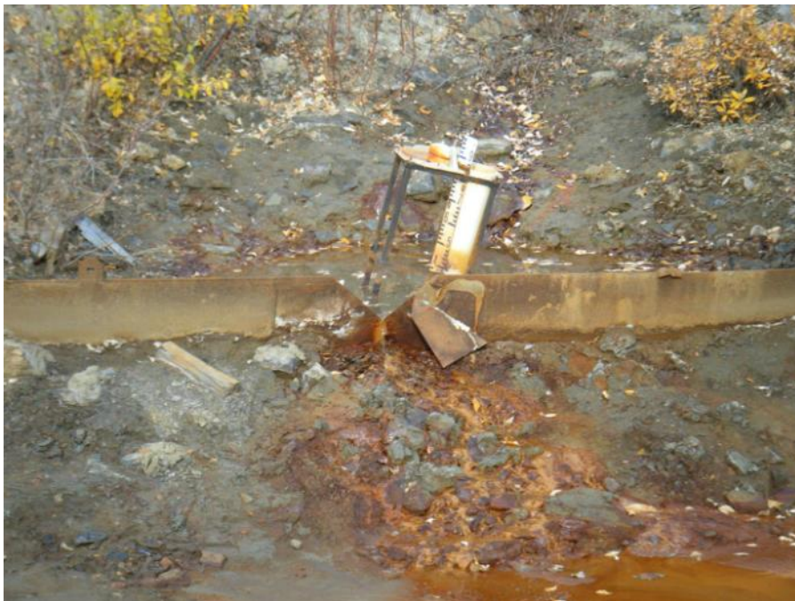
Photo 58 Vangorda Waste Dump Drain No. 3 weir - note delaminated weir plate and crooked staff gauge (September 20, 2011)
