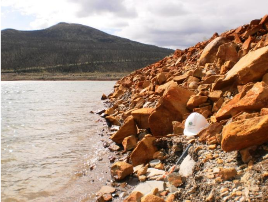
Photo 31 Wave erosion zone on upstream slope near pond level marked by hard hat and hammer (August 23, 2011)
