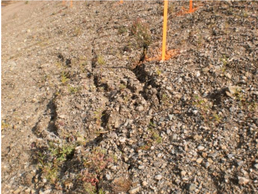
Photo 35 Close-up of horizontal cracks due to slope slump of surficial layer (August 23, 2011)
