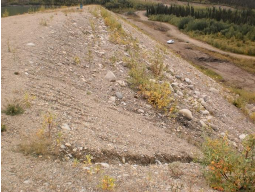
Photo 39 Crest and downstream slope of northeast portion of dam - note rill and gully erosion on slope (August 23, 2011)
