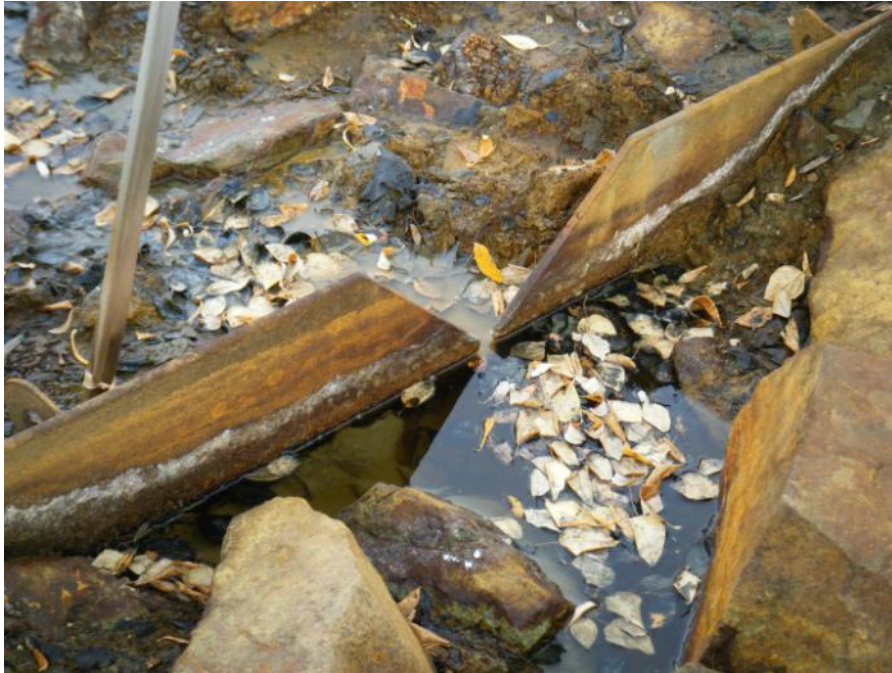
Photo 63 Vangorda Waste Dump Drain No. 5. Weir – weir plate split into two pieces at the V-notch (September 20, 2011)
