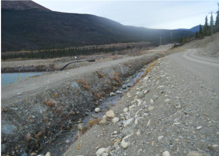
Photo 7 Lower reach of North Valley Wall Interceptor Ditch adjacent to Cross Valley Pond (September 20, 2011)
