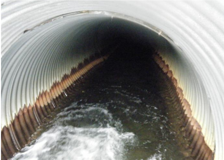
Photo 85 Upstream end of culvert to Vangorda Creek Diversion drop box - first pipe joint appears to be separated. (September 20, 2011)
