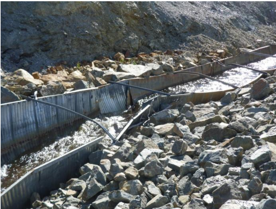
Photo 74 Battered section along lower reach of Vangorda Flume (May 30, 2012)
