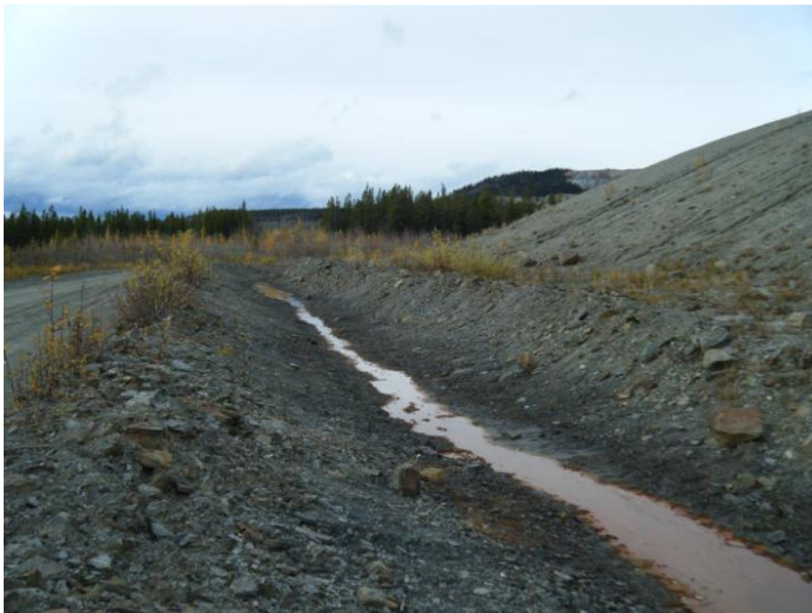
Photo 60 Vangorda Waste Dump Seepage Collection Ditch at Drain No. 3. looking downstream (September 20, 2011)
