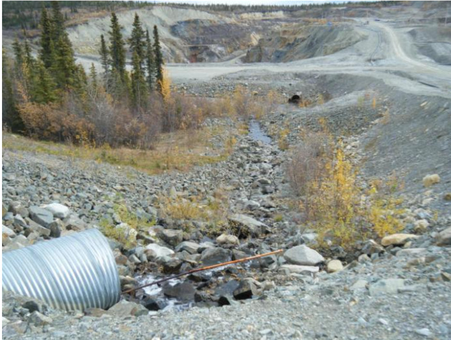
Photo 97 Culvert and ditch downstream of Sheep Pad Sediments Ponds weir - Vangorda Plunge Pool culvert in background (September 20, 2011)
