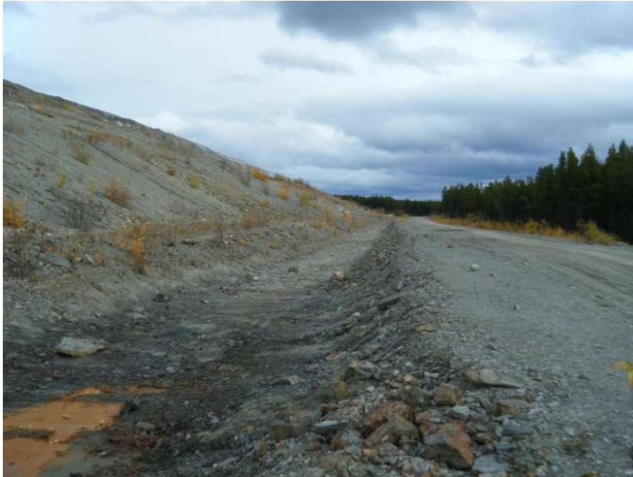
Photo 59 Vangorda Waste Dump Seepage Collection Ditch at Drain No. 3 - looking upstream (September 20, 2011)
