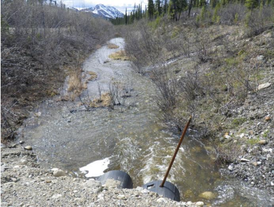
Photo 9 Channel downstream of Potable Water Well access road culverts - note sediment deposits at channel bottom (May 30, 2012)
