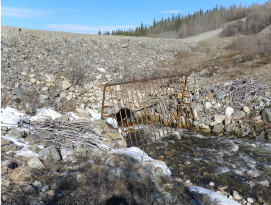
Photo 69 Vangorda Flume Diversion culvert inlet - note runoff entering into creek near culvert entrance (May 30, 2012)
