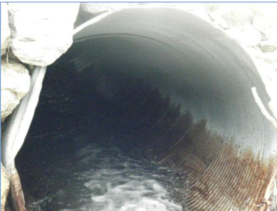
Photo 78 Upstream end of Vangorda Flume intake culvert - first pipe joint appears to be separated (September 20, 2011)
