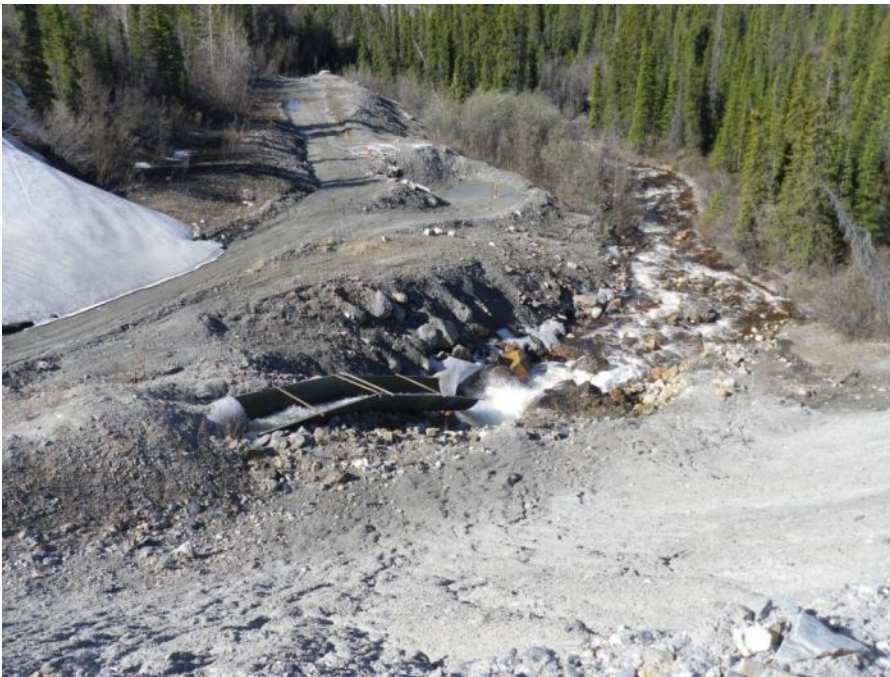
Photo 80 Discharge of Vangorda Flume flow via culvert leading from drop box as seen on Photo 79 (May 30, 2012)
