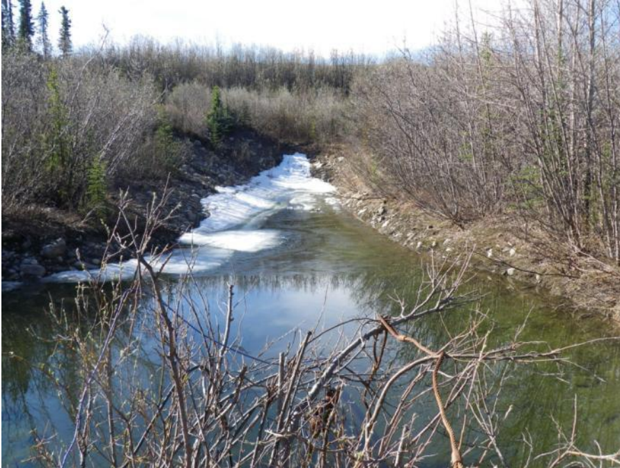
Photo 73 Excavated trench to collect surface runoff for pumping into Flume Diversion as seen in Photo 72 (May 30, 2012)
