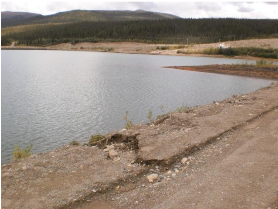
Photo 36 Gully erosion of downstream berm slope (August 23, 2011)
