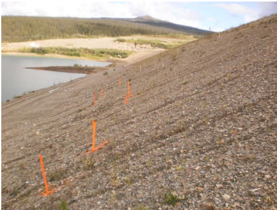
Photo 34 Rill erosion along downstream slope (August 23, 2011)
