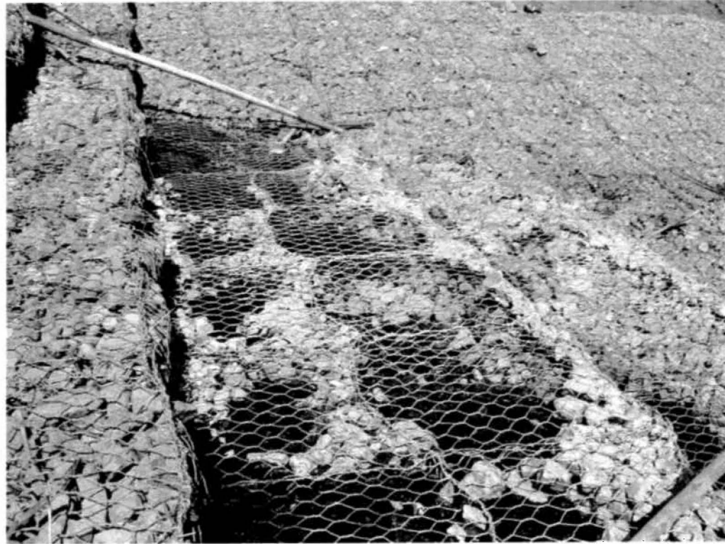
Photograph 1: Erosion of gabion fill from baskets following first spring freshet event
