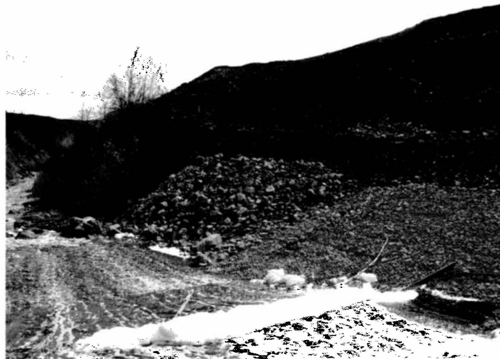
Photograph 5: Minimal erosion on right hand side of the channel transition downstream of Drop Structure 4.
