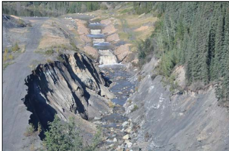
Figure 42 Clinton Creek Channel D/S of DS#4 on August 23, 2010
