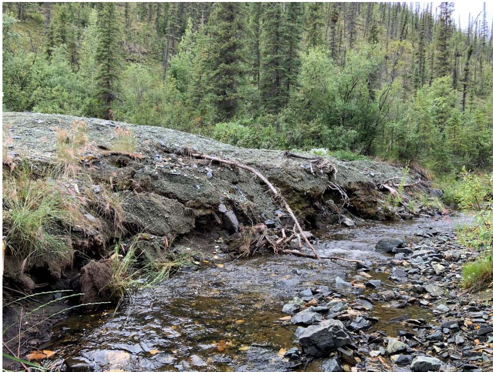
Appendix Photo 14. E3(H) – erosion along right downstream bank.
