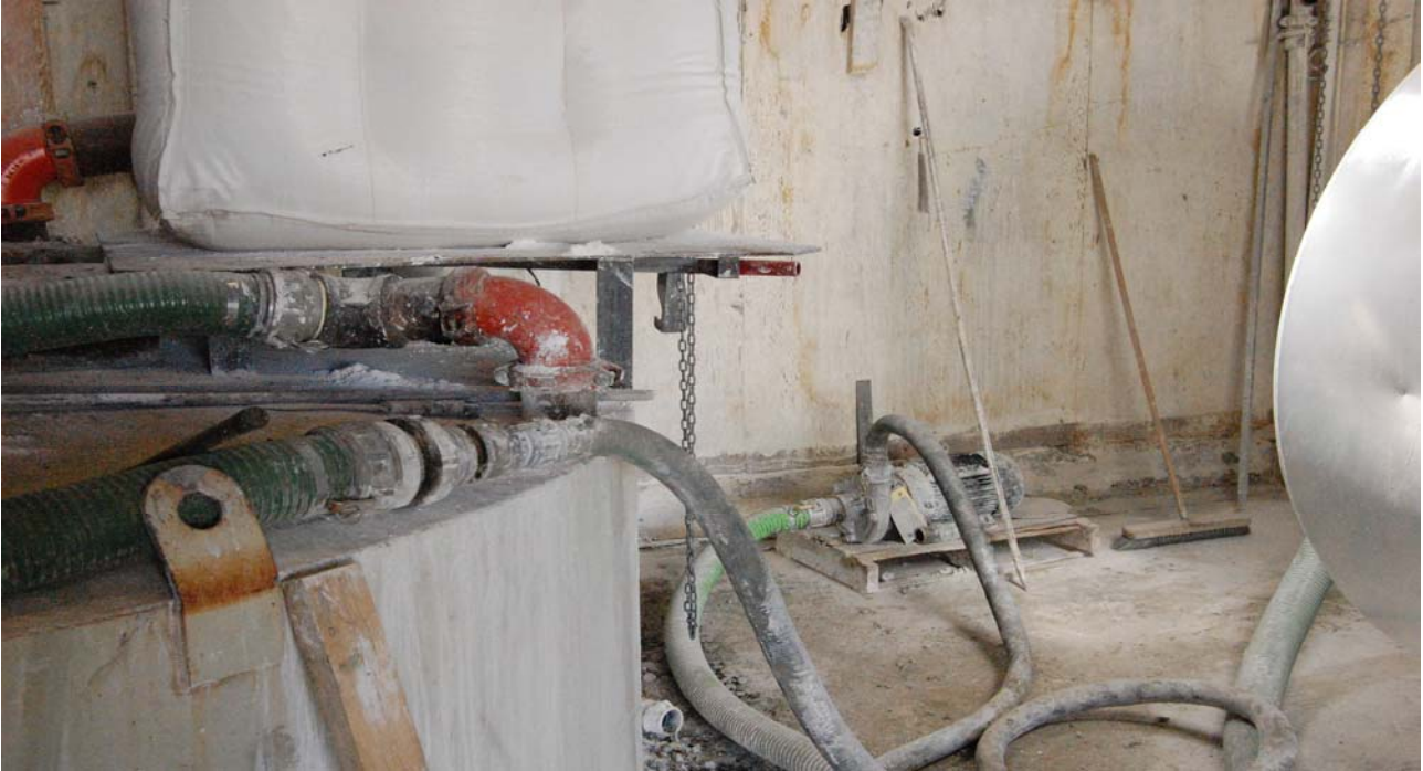
Figure 4: New Pump For Water Transfer From Water Storage Tank To Lime Mixing Tank
