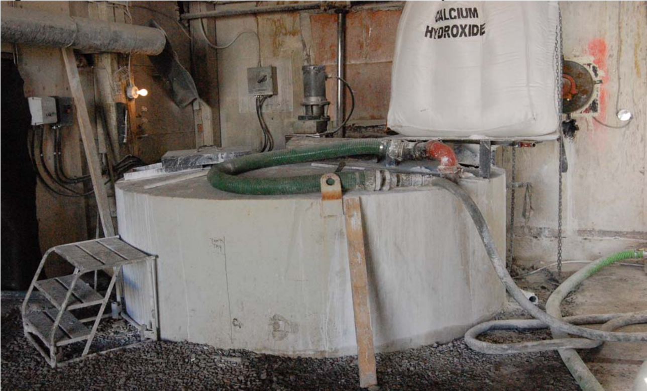
Figure 3: In-Ground Tank To Increase Ease Of Use And Safety Of Workforce
