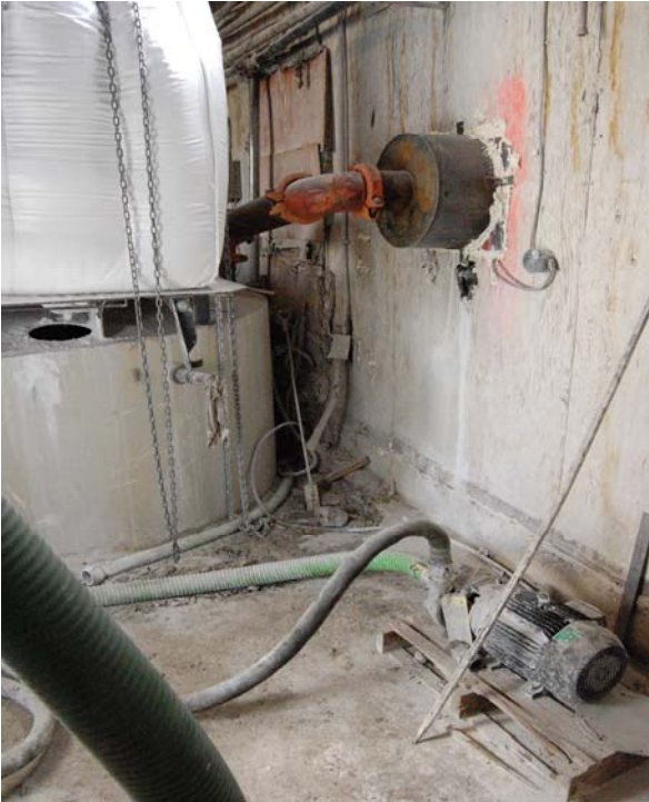
Figure 6: Safety Platform and Shut-off Latch, In-ground Lime Mixing Tank, Centrifugal Pump, and Exhaust Fan
