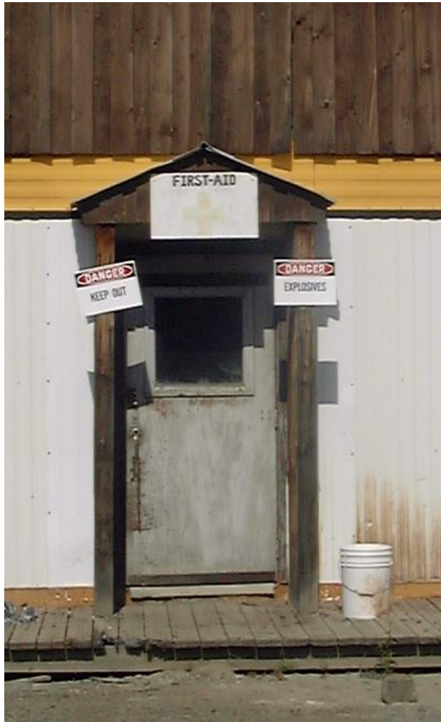
Fig. 3 – First Aid building at Elsa Townsite, with explosive hazard identified and door locked.
