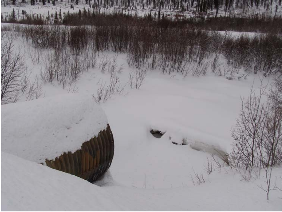
Photo 3 – Perched culvert at Rose Creek crossing.
