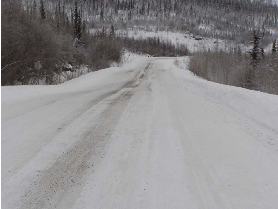
Photo 2 – Access Road. and typical road settlement.
