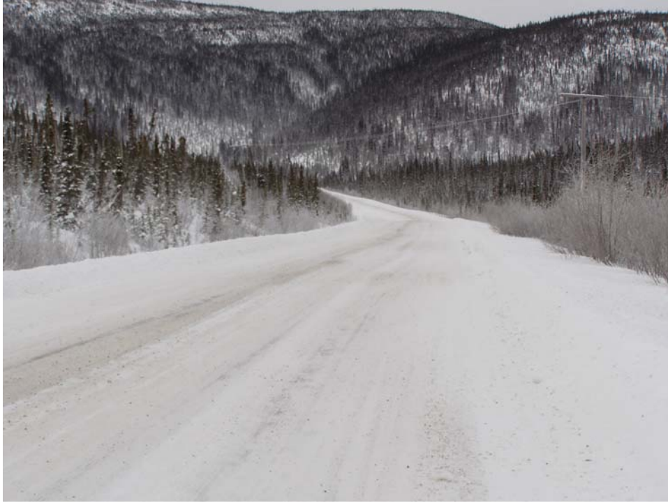
Photo 1 – Access road from Faro to mine site showing typical road settlement.
