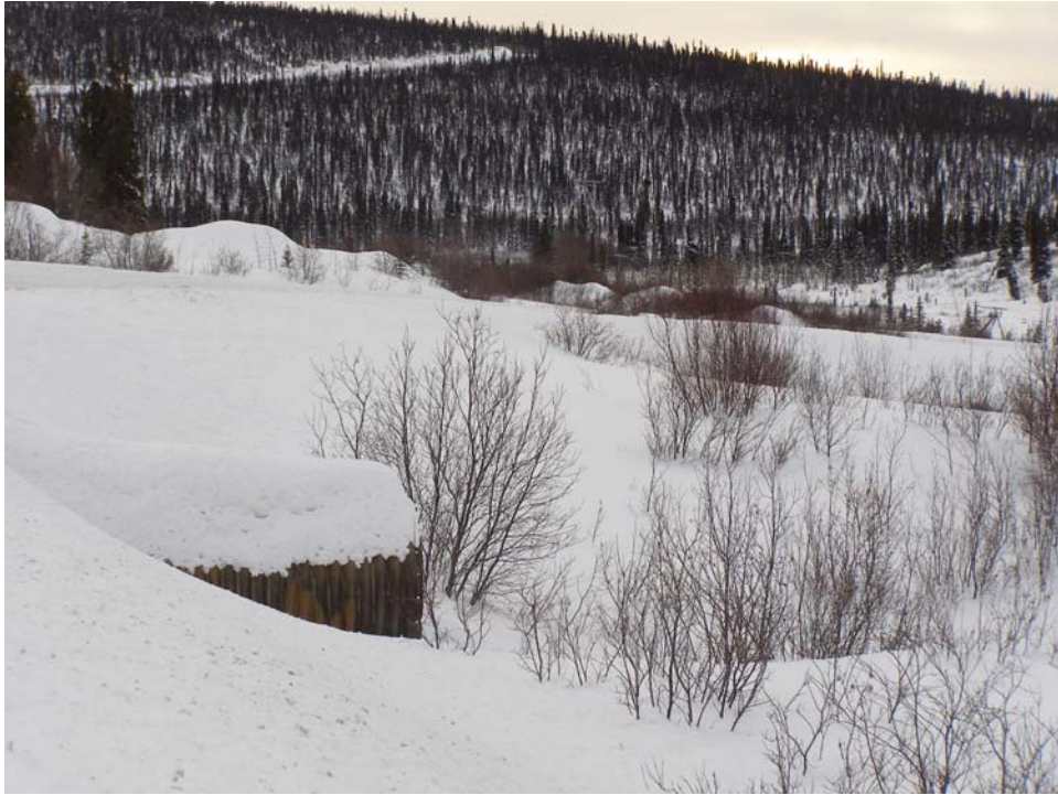
Photo 4 – Other end of perched culvert.
