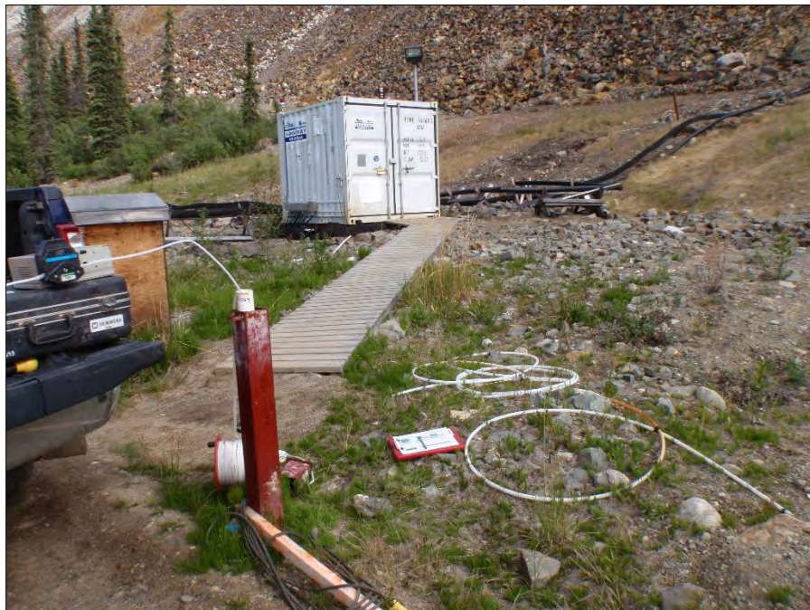
Photo 20: View of well P09-SIS4. Photo taken on June 15, 2015.
