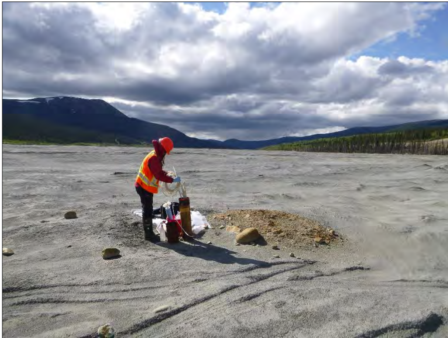
Photo 22: View of CMT wells P03-06-1, P03-06-2, P03-06-6 and P03-06-7. Photo taken on June 11, 2015.
