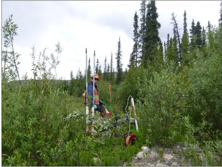
Photo 37: View of well SRK05-5C. Photo taken on June 12, 2015.
