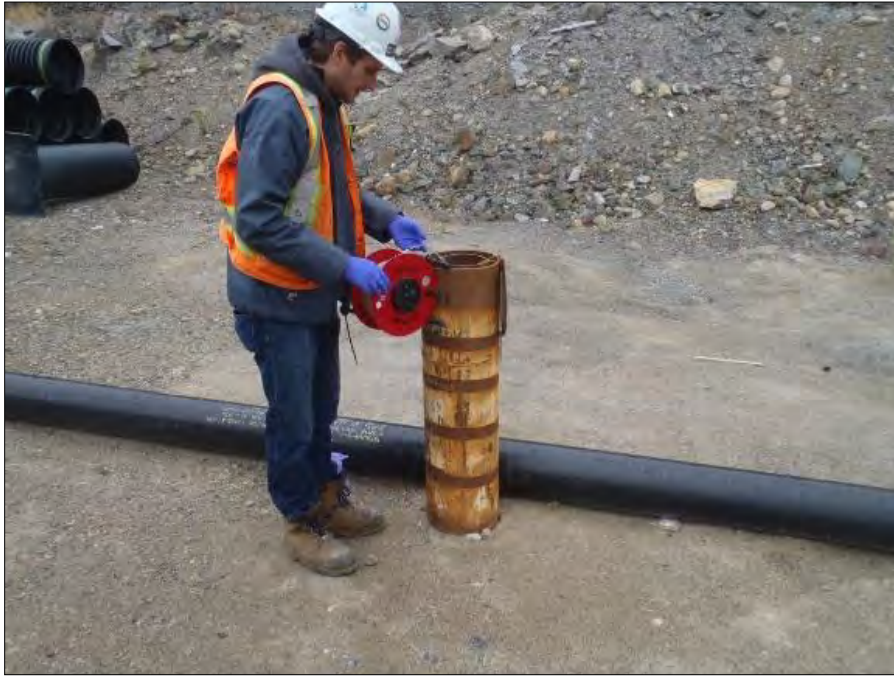
Photo 47: View of well PW14-06. Photo taken on June 10, 2015.
