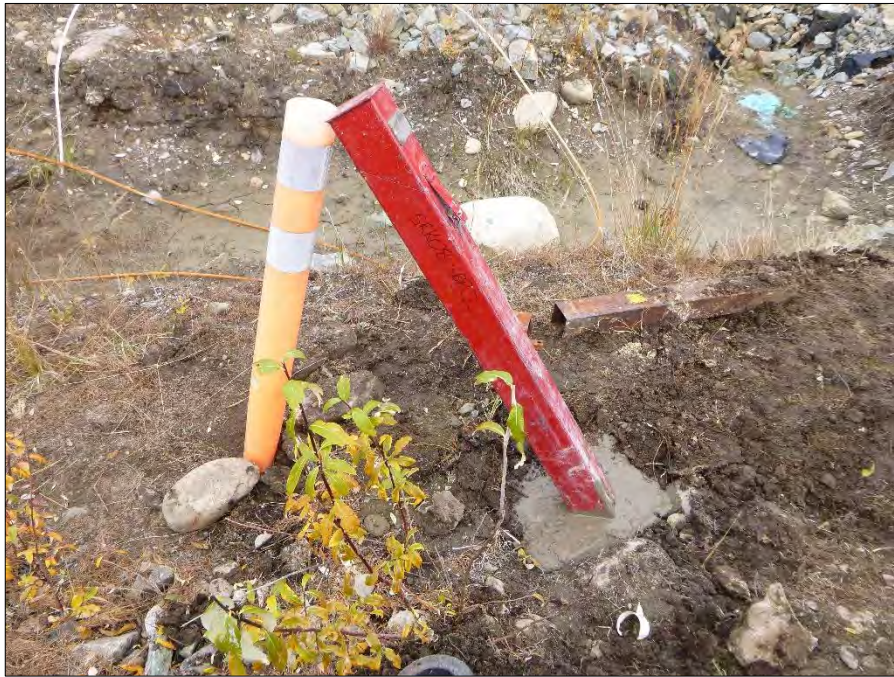
Photo 99: View of well SRK08-SBR2. Photo taken following well repairs on September 14 th , 2015.
