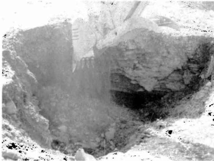
Photo 8: Excavator starting to fill collapsed stope.
