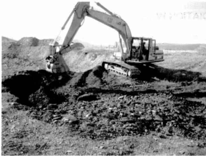
Photo 9: Collapsed stope nearly filled to completion.
