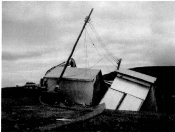
Photo 2: View of Shamrock J building partially collapsed over open vent raise.
