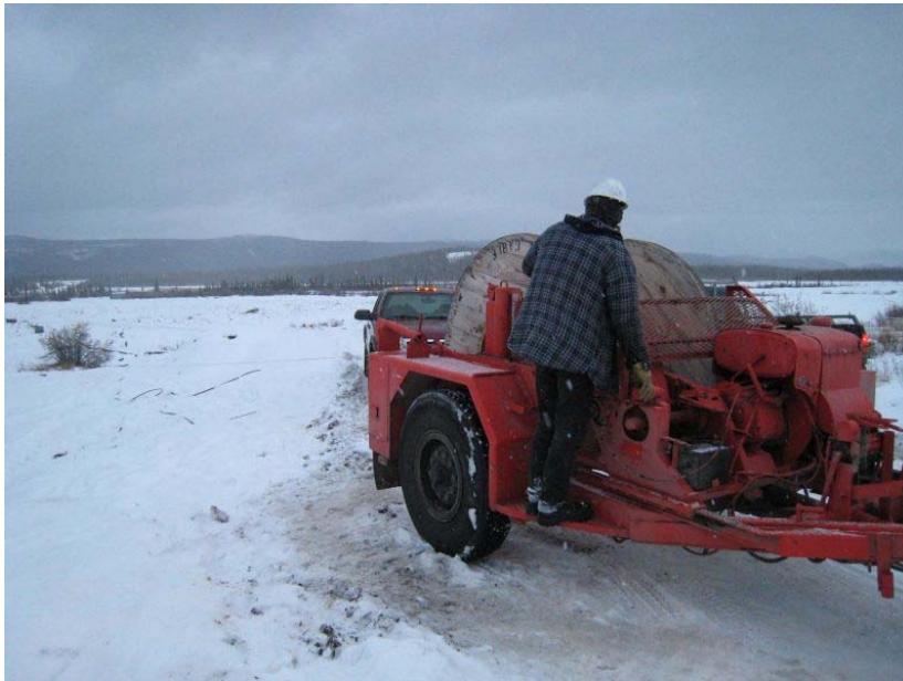
Photo of personnel operating wire spooler in the Framing Yard to Tailings Area section
