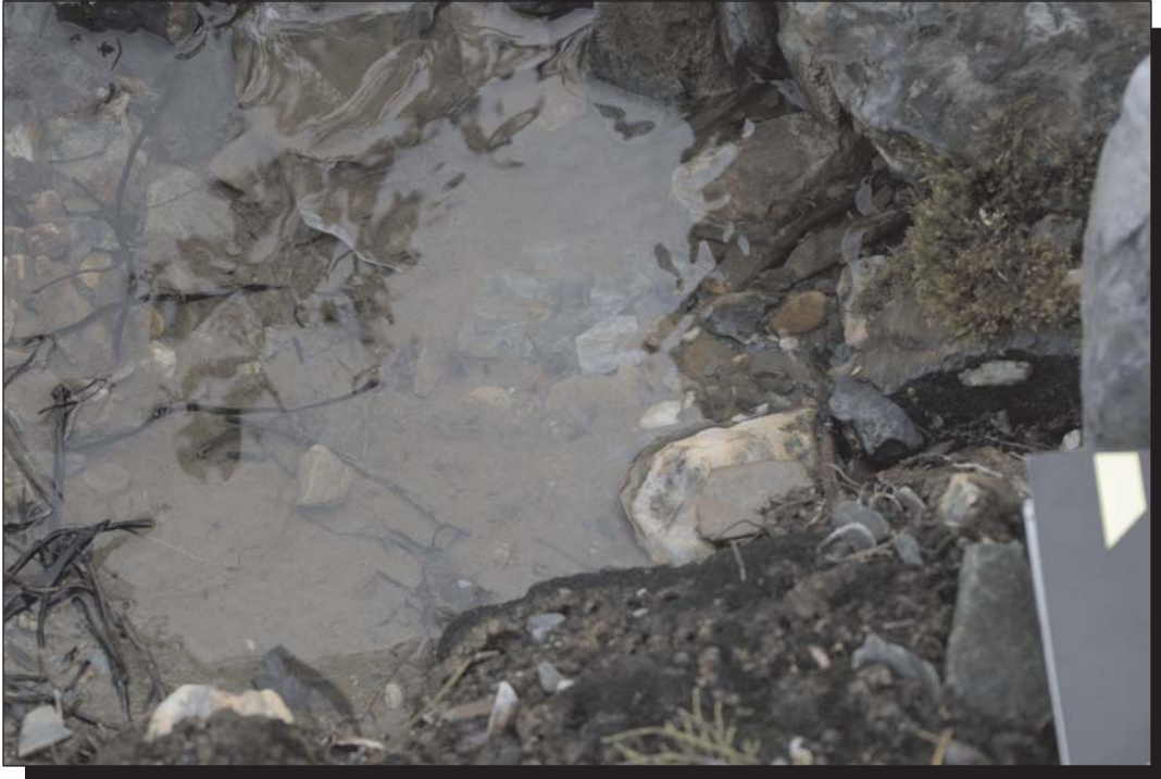
Photo 5 Sand present in seepage location at toe of North Dam. Photo taken Aug. 6, 2008
