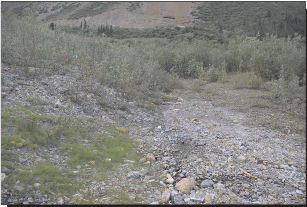
Photo 4 Soft/seepage area at toe of North Dam. Aspect: NW. Photo taken Aug. 6, 2008
