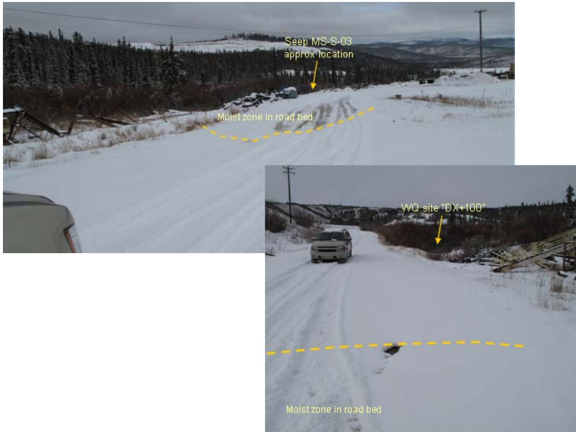
Photo 4. Moisture zone on access road to lower mill platform, October 18.
