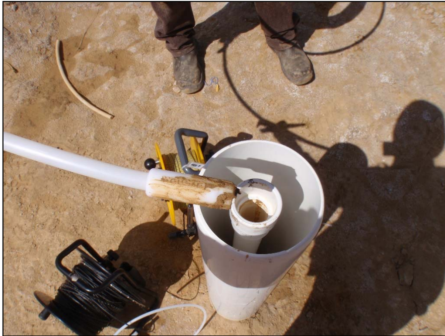
Photo 51: View of well MW09-01. Unable to get any more tubing into well due to large amount of soil found on waterra tubing already existing in well. Photo taken on June 27 th , 2014.
