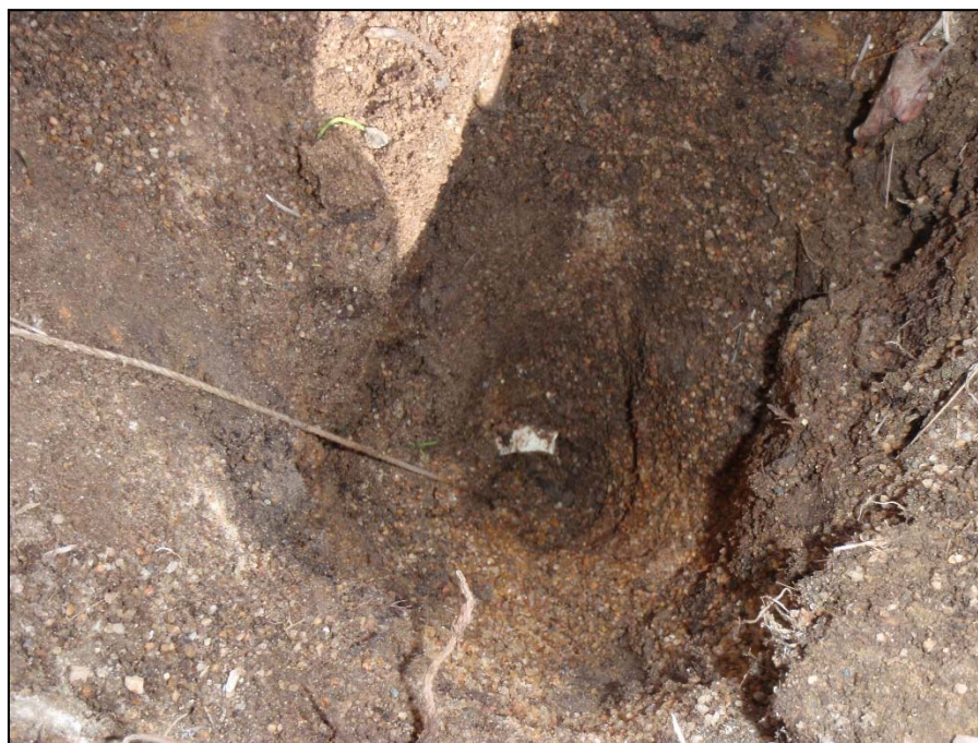
Photo 16: View of damaged well MW09-17. Existing bailer stuck in well due to large amount of soil that had fallen into well. Photo taken on June 26 th , 2014.
