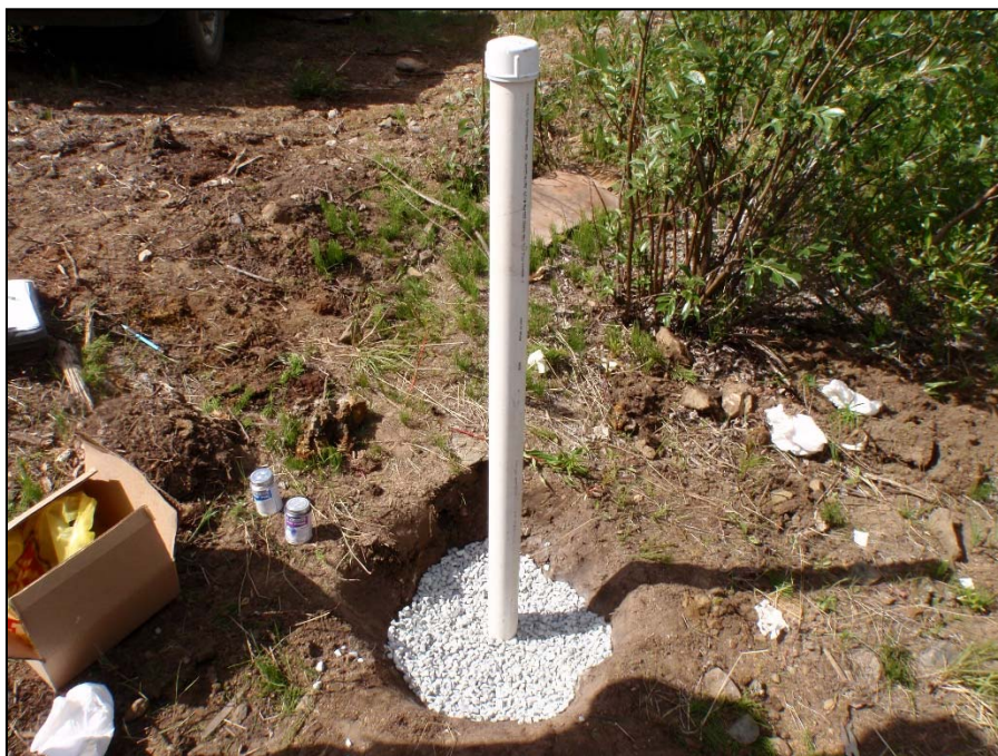
Photo 19: View of the third step during well repair for well MW09-17. Bentonite chips were used to seal the previously dug hole around stick-up. Photo taken on June 28 th , 2014.
