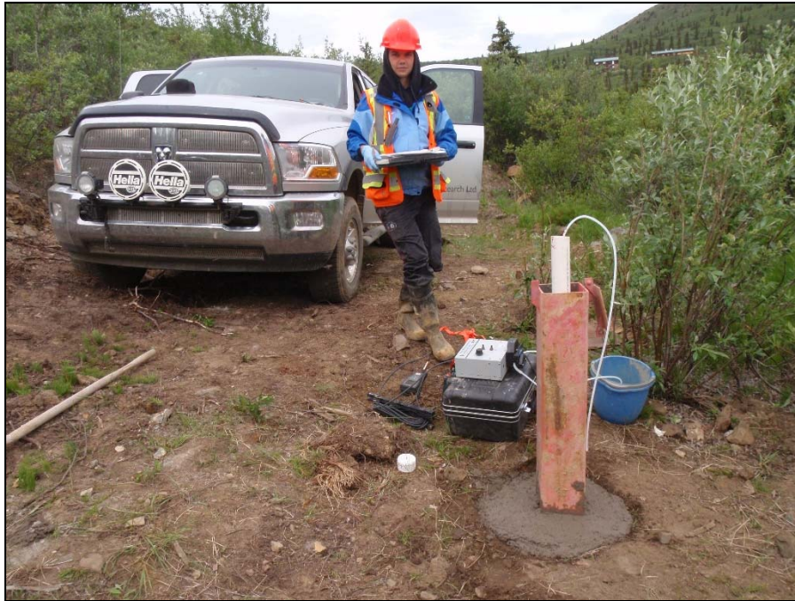
Photo 21: View of the fifth step during well repair of well MW09-17. The steel monument was replaced around the PVC well with concrete. Photo taken on June 29 th , 2014.
