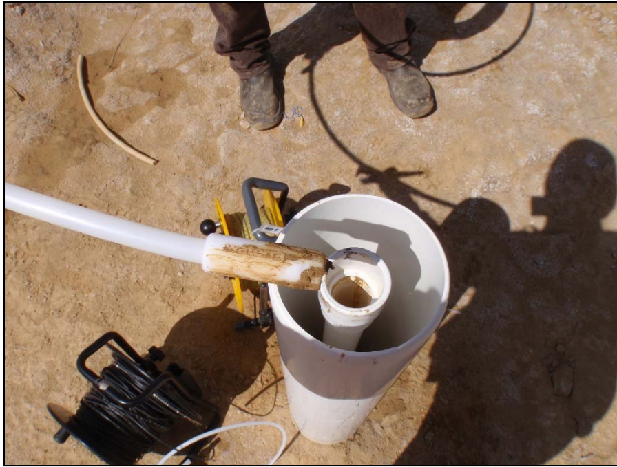
Photo 51: View of well MW09-01. Unable to get any more tubing into well due to large amount of soil found on waterra tubing already existing in well. Photo taken on June 27 th , 2014.
