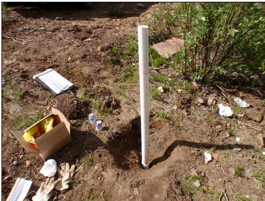
Photo 18: View of the second step during well repair for well MW09-17. A cup-link and new PVC pipe were attached. Photo taken on June 28 th , 2014.
