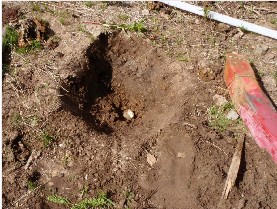
Photo 17: View of the first step of well repair for well MW09-17. A hole was excavated around well to the top of where the stick-up was broken. Photo taken on June 28 th , 2014.
