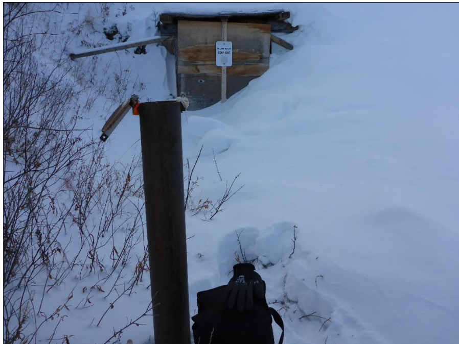
Photo 24: View of well GLL07-02. Photo taken on February 1, 2017.
