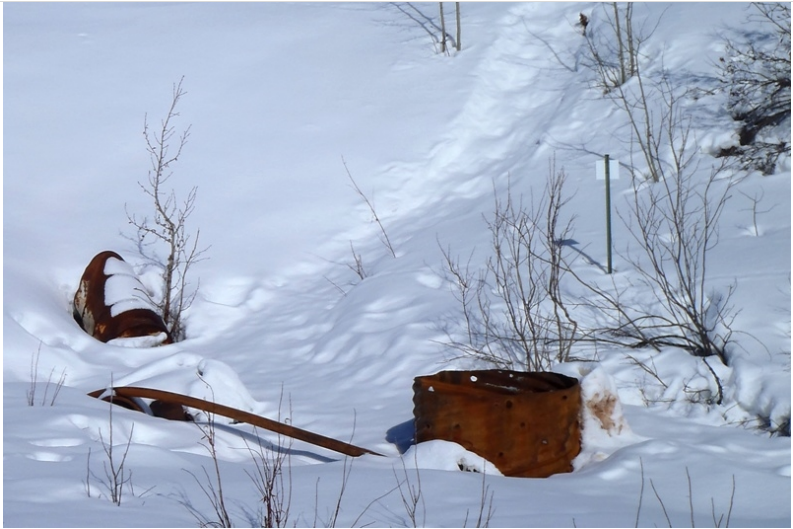
H/WQ-SEEP pipe was not secured to the culvert at the time of site visit. Sampling crew temporarily affixed it but more robust connections are recommended.
