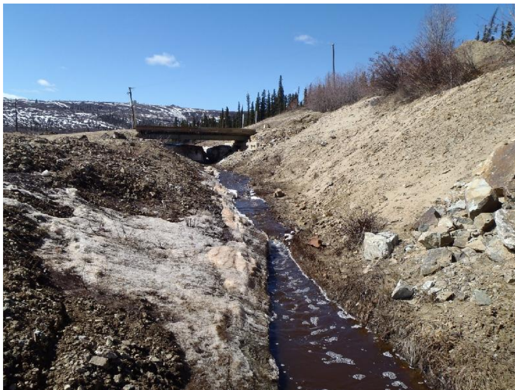
Photo 8. H-DC-DCB looking upstream. Small quantities of snow and some ice remain along north-facing channel slopes.
