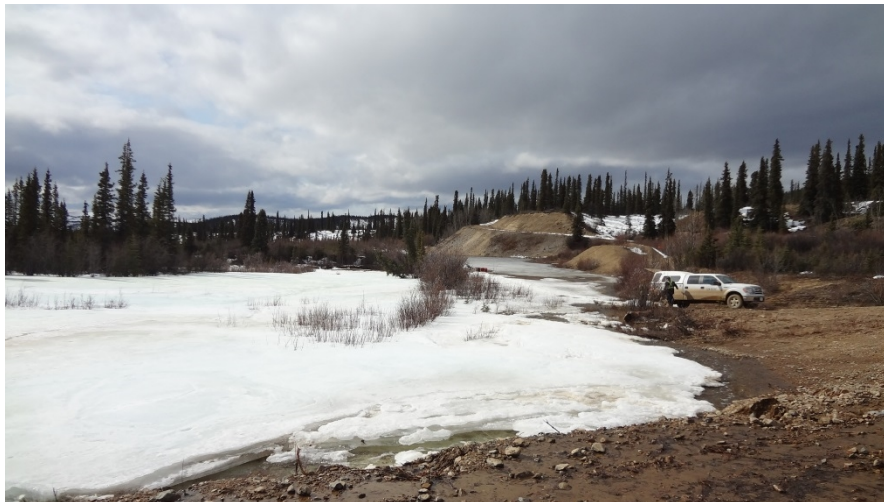
Photo 15. H-VC-R from road. Water flowing out of second culvert, ponding in parking area.
