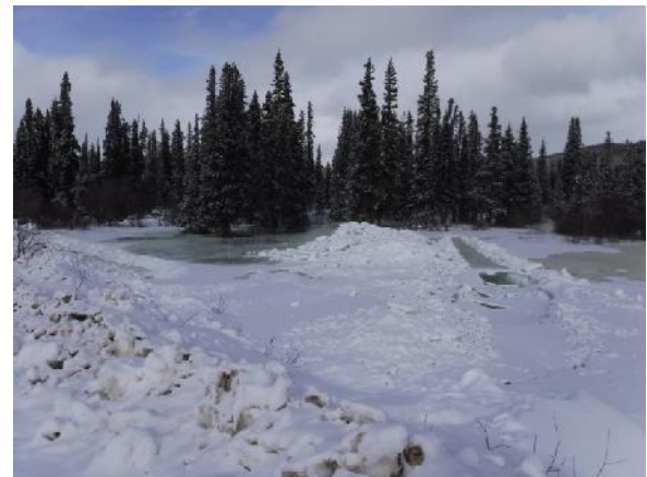
Photo 18. Upstream of road crossing at Victoria Creek (H-VC-R). View of overflow ice and excavation work.
