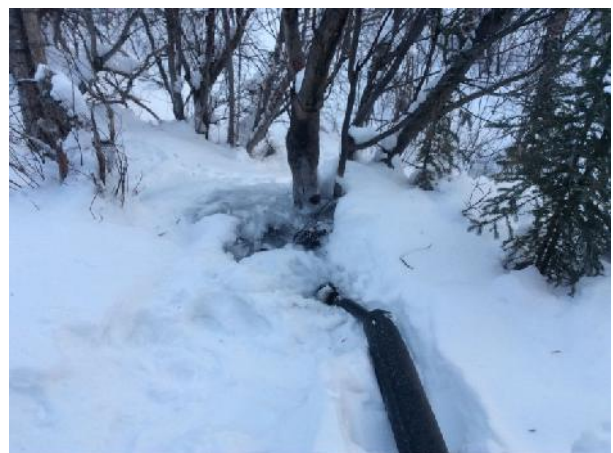
Photo 22. WQ-PW – pipe outlet.
