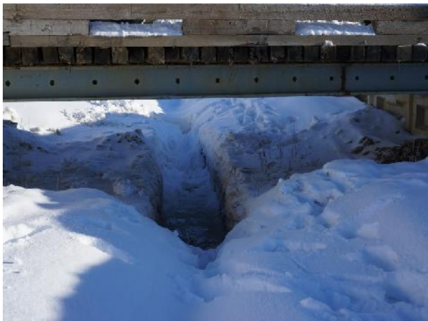
Photo 3. H/WQ-DC-B – looking upstream (stagnant water at site).
