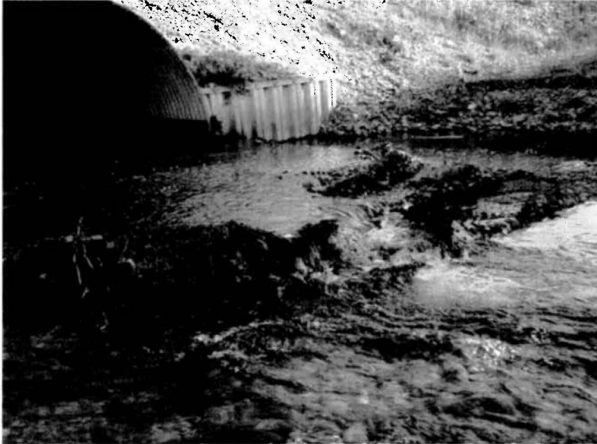
Figure 3. Gabion baskets appear to have shifted from the location at which they were originally placed. Baskets have been pushed up and out of the water in several spots. Baskets have also become filled with debris.
