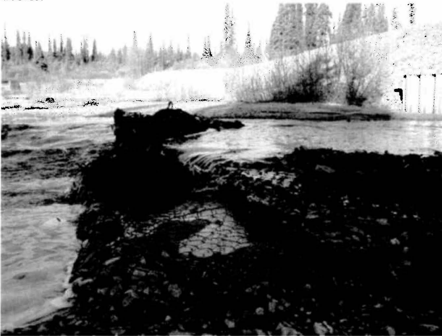
Figure 4. Much of the rock material appears to have been washed out of the gabion baskets since their construction.
