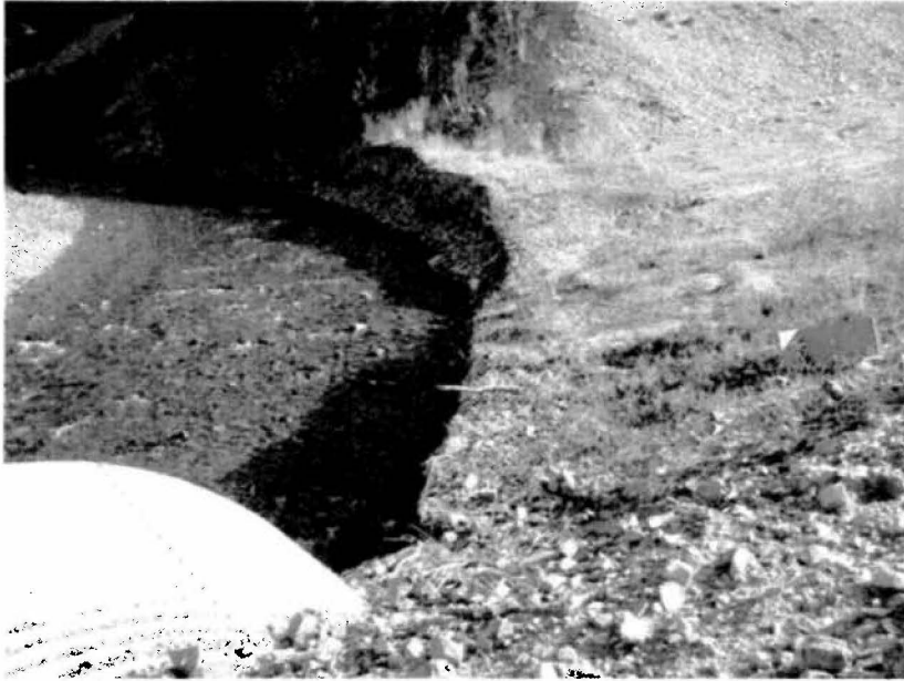
Figure 1. Gabion baskets were installed on the left-hand side of the stream (river-left) presumably as an erosion protection device. Baskets installed at this location appear to have been effective in preventing bank erosion adjacent to the culvert. Erosion of the left bank upstream of the baskets is occurring.
