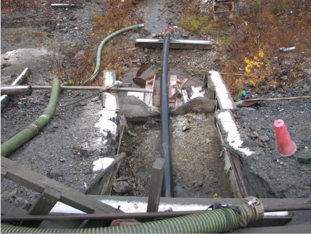
Downstream side of dam 2 outlet structure. Note poor condition. Siphon hose in place
