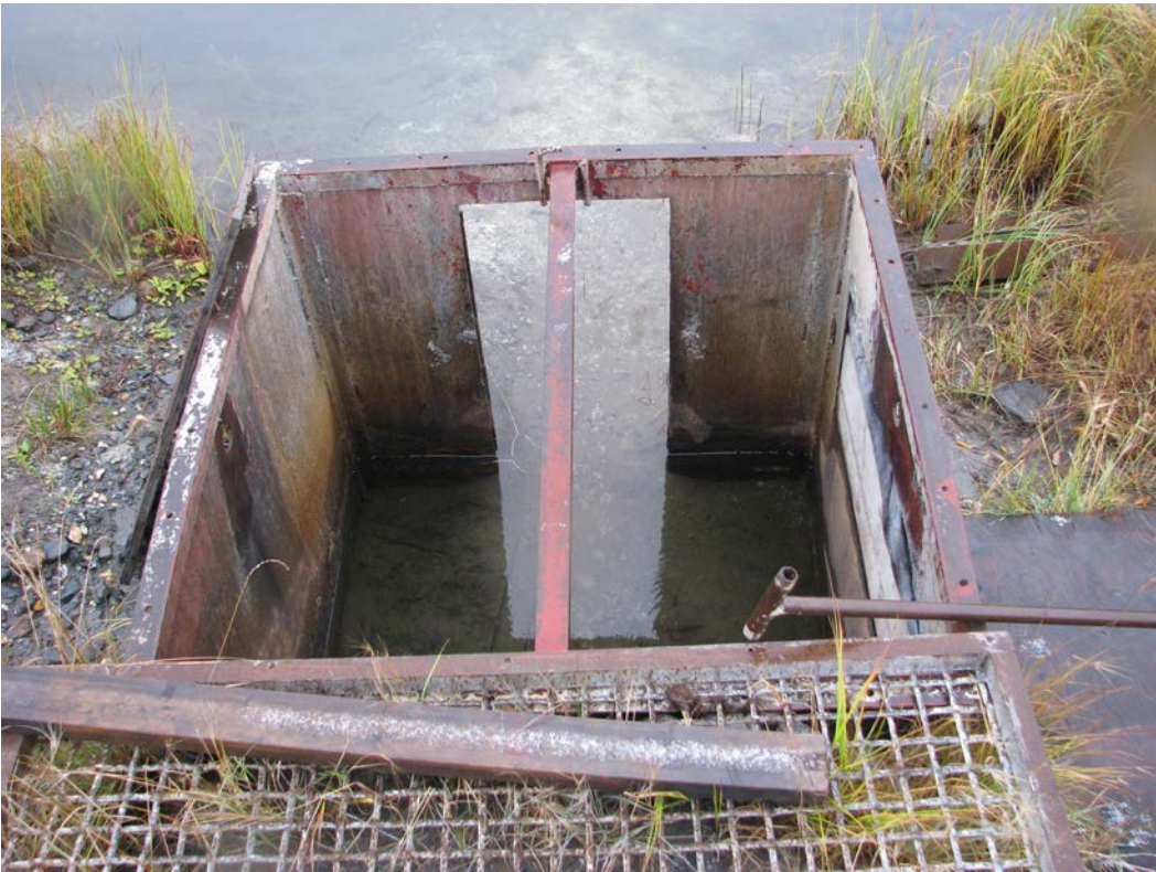
Dam three outlet structure. Upstream side
