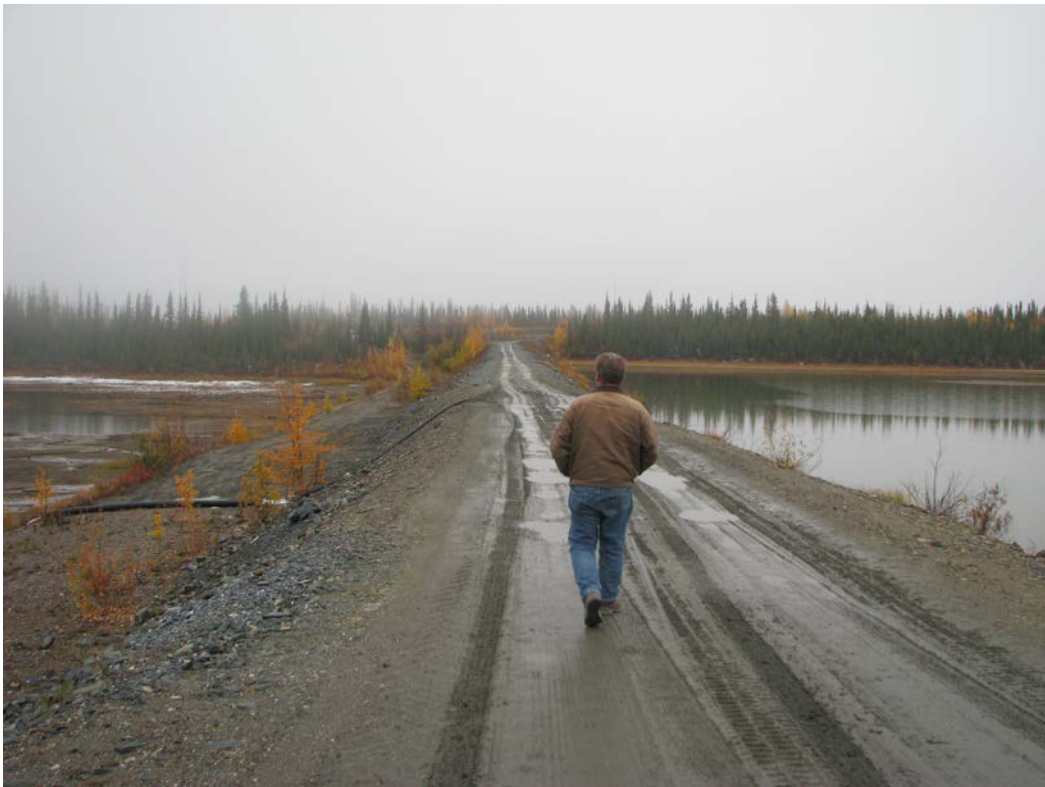
Crest of dam 1. Note low area of crest ahead of Frank Patch. Siphon hose can be seen
