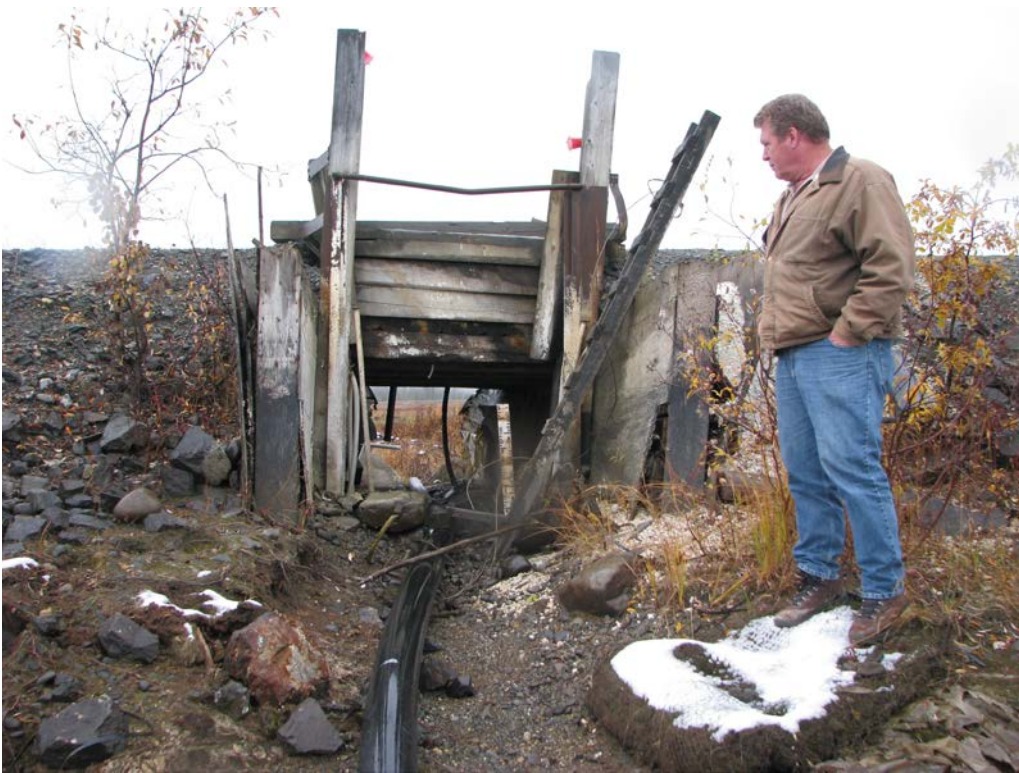
Frank Patch at D/S side of outlet structure Dam 2
