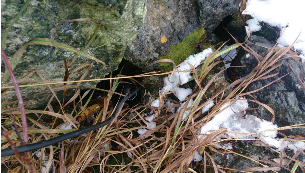
Photo 29: Site GWCC-1—Seepage from rock dump to ponded area of Porcupine Creek.
