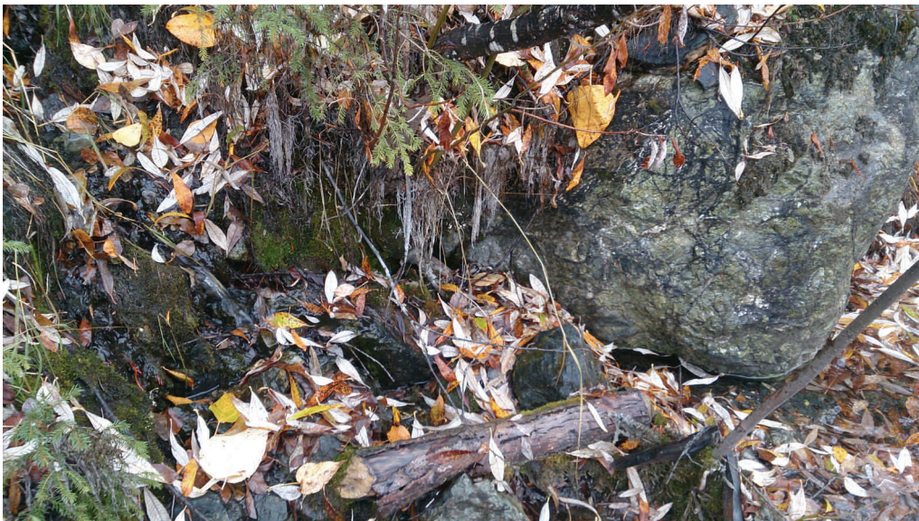
Photo 36: Site GWCC-4—Seepage from Rock dump into side channel.
