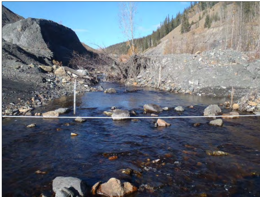
Photo 7: Upstream view of relocated Site E1 (Clinton Creek downstream of gabions). Photo taken on September 19, 2014.
