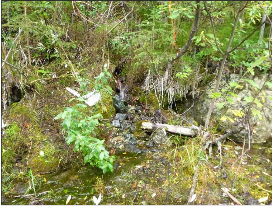
Photo 19: View of groundwater seepage Site GWCC-3. Photo taken on July 26, 2015.
