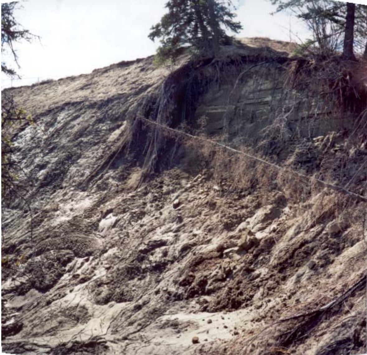
Photograph 9. May 2002. Active sloughing at thawing silt at contact with capping eolian sand within the Steele Street Slide headscarp.
