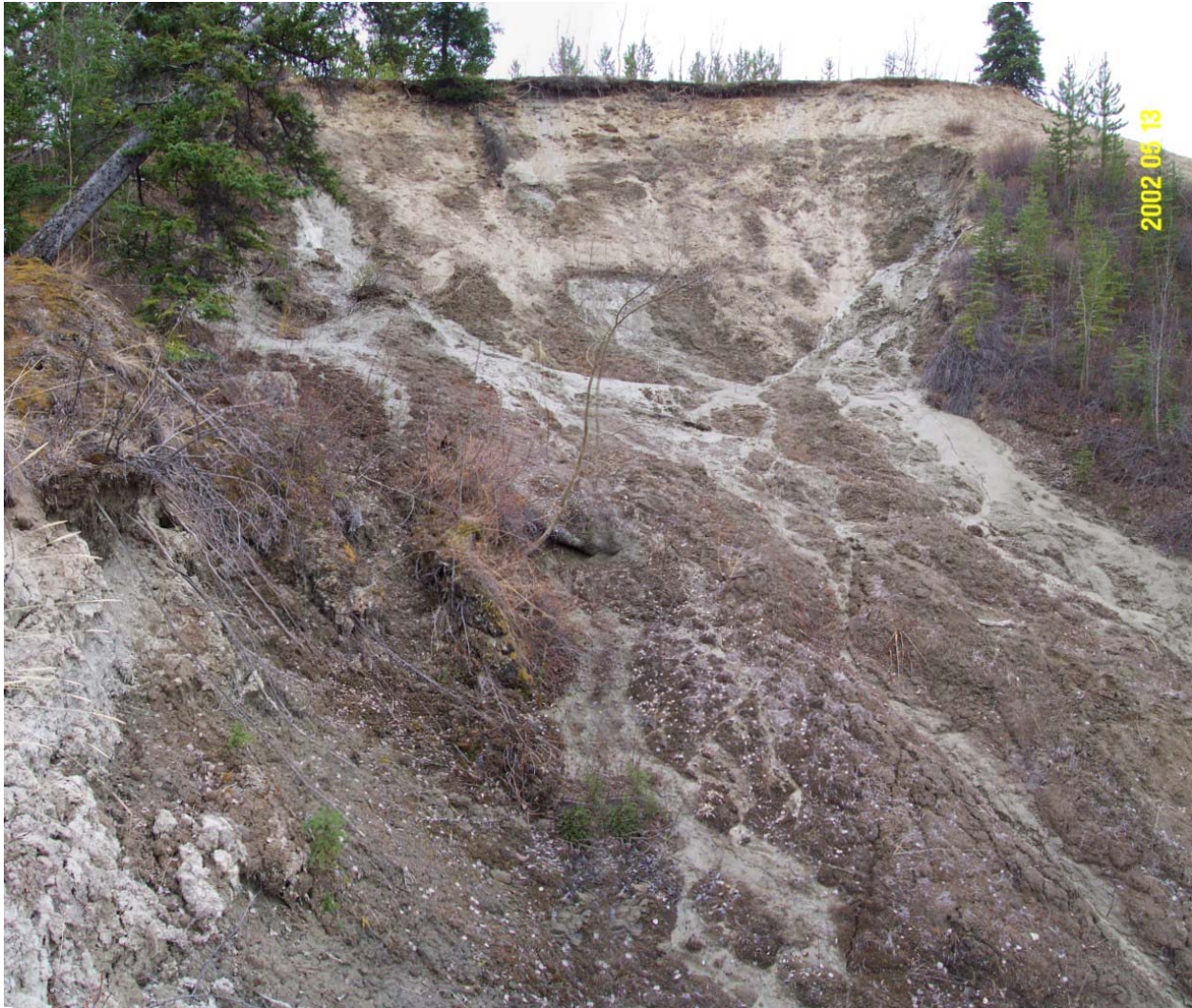
Photograph 6: May 2002. Headscarp of an active area of thawing saturated silt below the eolian sand on the Lambert Street Slide. Detail of the specific active areas is shown on Photographs 7 and 8.
