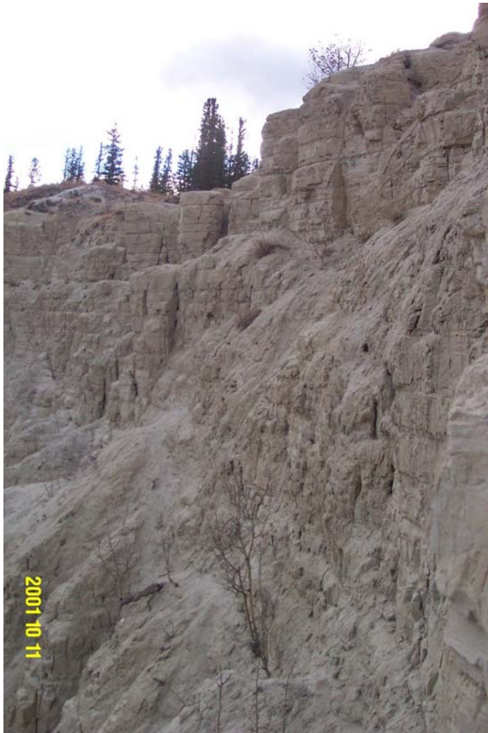
Photograph 16: May 2002. Sub-vertical bluffs of compact silt on the upper escarpment slopes above the end of Baxter Street
