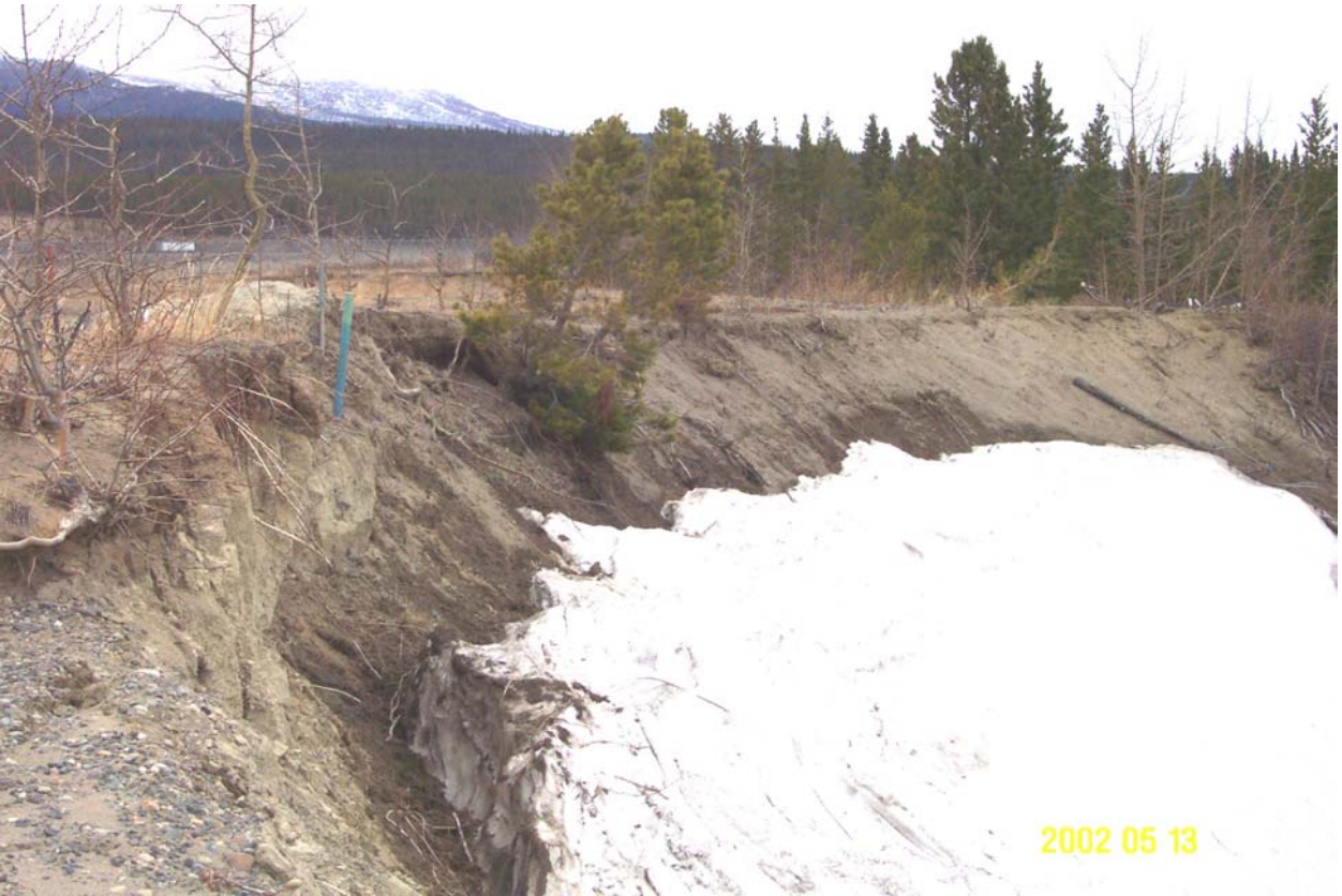
Photograph 4: May 2002. Main Street Slide. Melting snow in the headscarp contributes to the erosion process. The blue pipe stem to the left of centre is the slope stability indicator casing installed in 1970 and used for this study.
