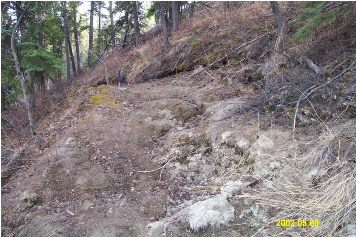
Photograph 13: May 2002. Tension crack formed upslope of the headscarp of the Takhini debris slide.
