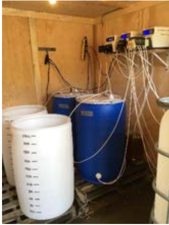
BRs inside the shed
