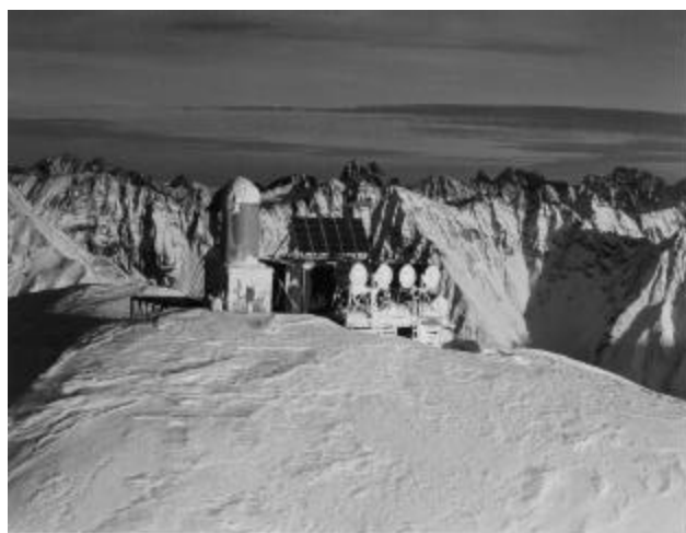
Figure 1. NorthwestTel Solar PV-Diesel Powered Microwave Radio Repeater
