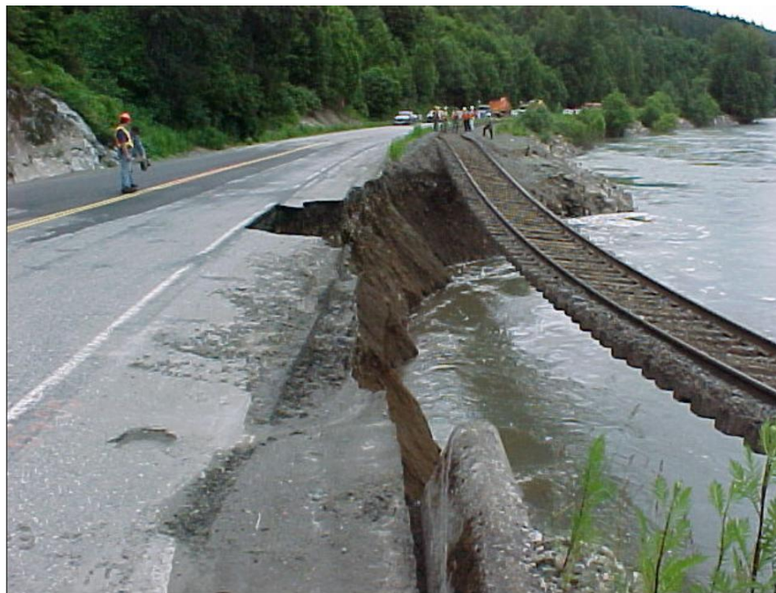
Picture 23: Inadequate Erosion Protection
