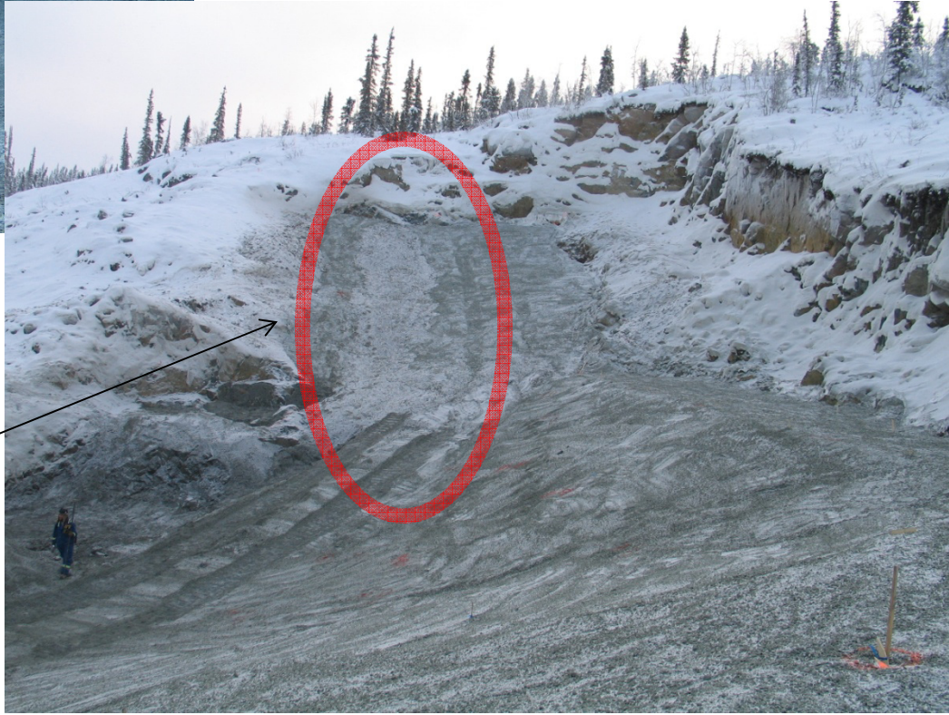
A zone of tailings mixed with bentonite was used to create a low permeability zone between the liner system and the bedrock surface
