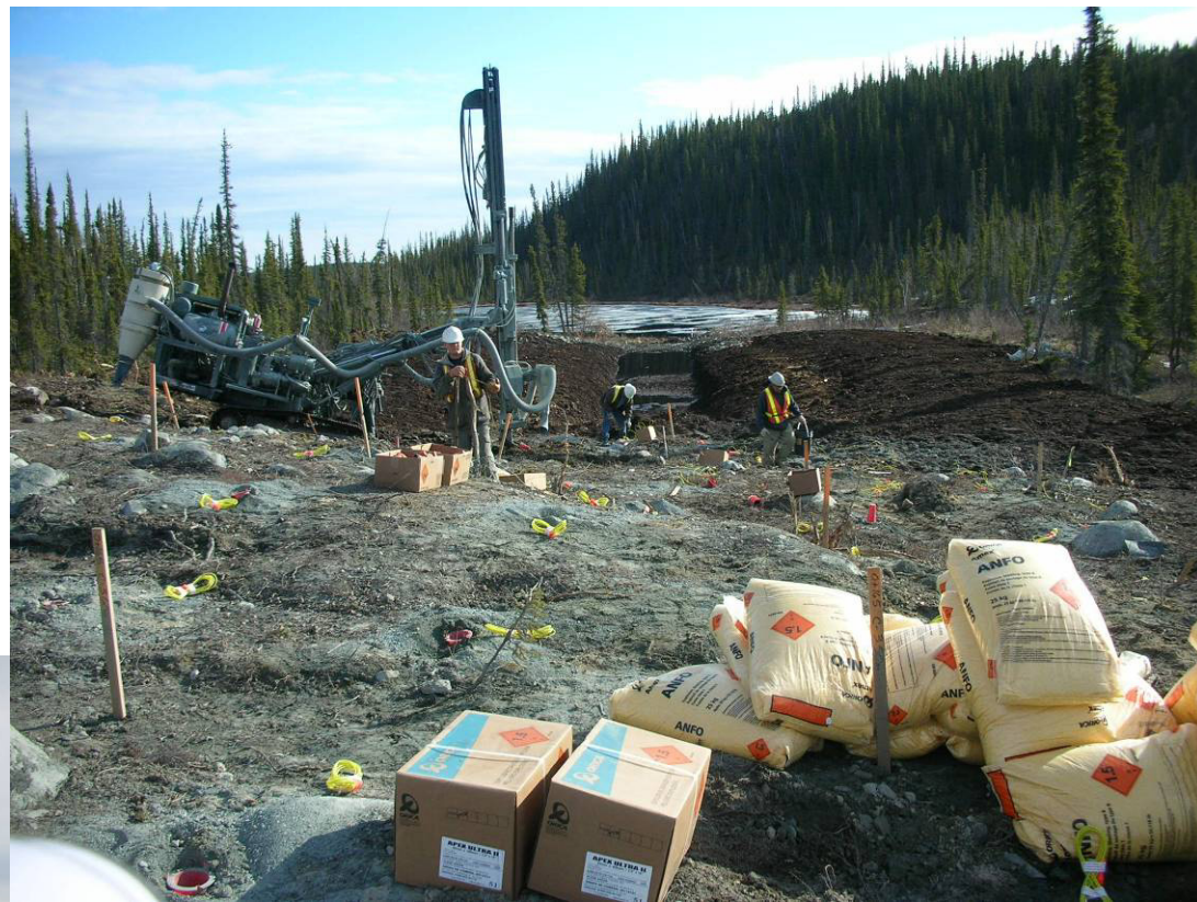
Excavation of peat and blasting of bedrock along the downstream reach of the Discharge Channel
