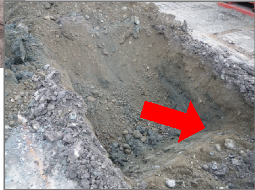
Note the staining in shallow soil
