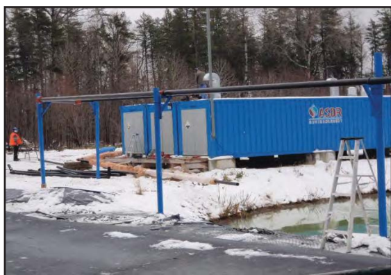
Picture 4. ASDR treatment units on site
