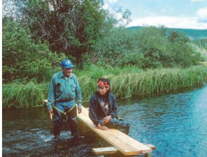
Dan Van Bibber and Eugene Alfred building a footbridge over Daghwát Tagéá (Mica Creek), 1991.
