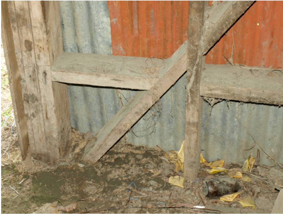
18. Exterior Photo: Water Damage
