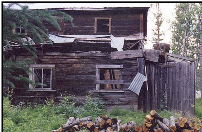
Southeast Corner and Building Interior, As Found Condition, June, 2002
