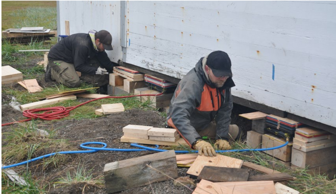
Gisli Balzer (left) Stephan Biederman (right) placing wooden shims under the building in August 2023.
