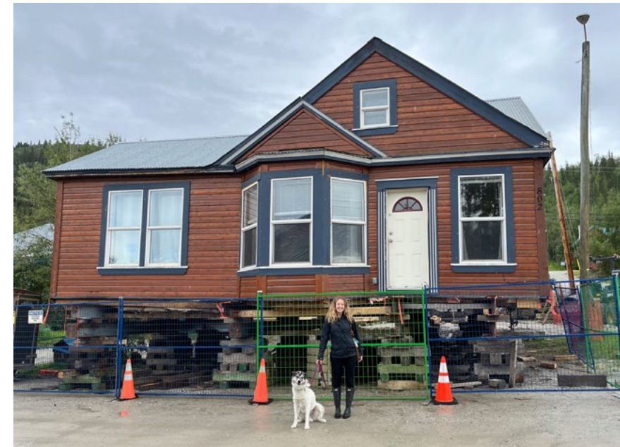
Karen Murray and her dog, Arrow, in front of the house when it was sitting in the middle of the street while the basement was being filled in.
