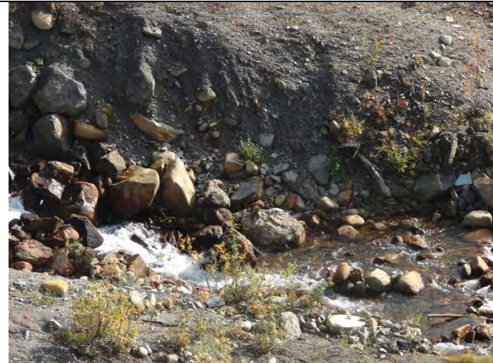
Photograph 4: Looking at the unprotected banks on one side of the Plunge Pool – 09-11-2013
