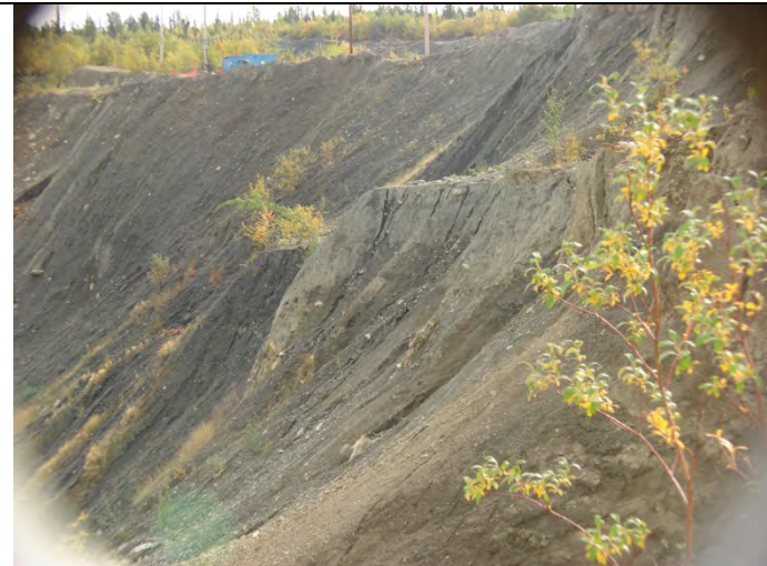
Photograph 40: Looking at Vangorda Pit side walls, showing rock raveling and slumping failures (6) – 09-10-2013
