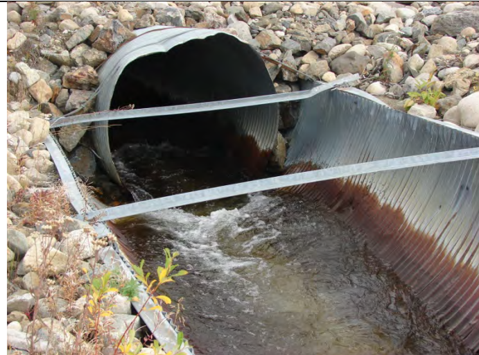
Photograph 34: Looking downstream of existing 1,500 mm CSP culvert and upstream of half-round 2,400 diameter CSP Culvert on existing VCD – 09-10-2013
