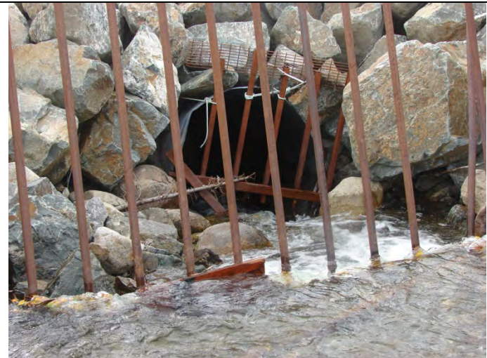
Photograph 32: Looking at the existing 1,500 mm culvert inlet on Vangorda Creek north of access road (2) – 09-10-2013
