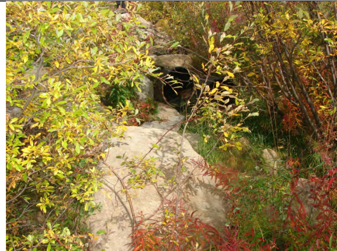
Photograph 18: Looking at the culvert outlet on existing channel west of SRK proposed alignment, between station 1+000 and 1+1050 (4) – 09-10-2013
