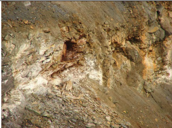
Photograph 35: Looking at Vangorda Pit side walls, showing rock raveling and slumping failures (1) – 09-10-2013
