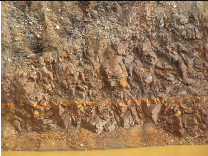
Photograph 37: Looking at Vangorda Pit side walls, showing rock raveling and slumping failures (3) – 09-10-2013
