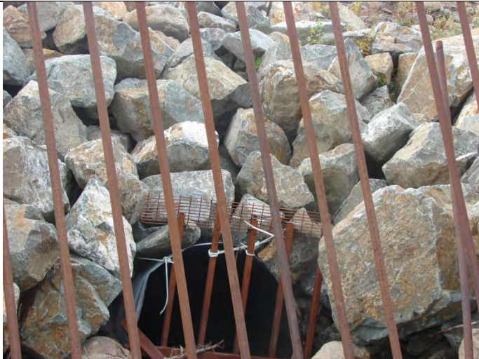
Photograph 33: Looking at the existing 1,500 mm CSP culvert inlet on Vangorda Creek north of access road, large rock riprap (3) – 09-10-2013
