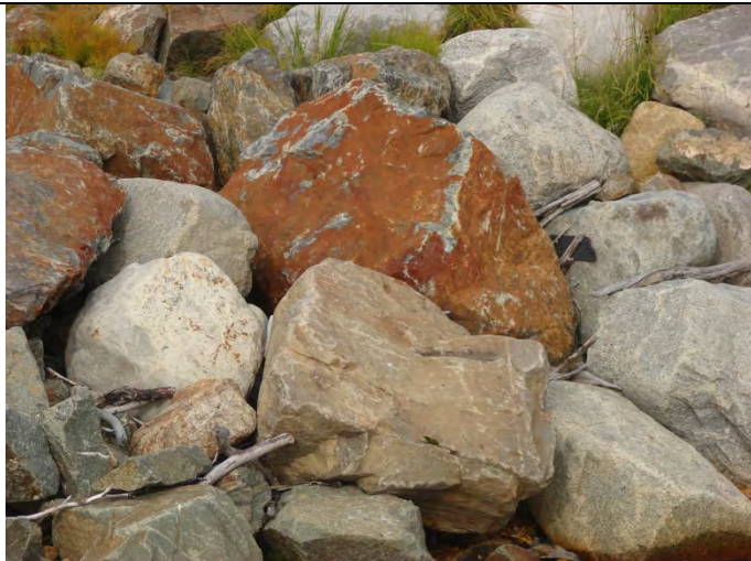
Photograph 11: Looking at large sized rock placed at the Plunge Pool, at station 1+1300 – 09-10-2013
