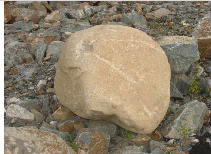
Photograph 12: Looking at large sized rock at Plunge Pool estimated at 1.5 m diameter, at station 1+1300 – 09-10-2013
