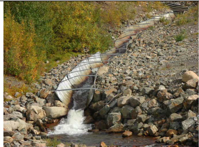
Photograph 8: Looking half-round 2,400 diameter CSP Culvert discharging to plunge pool at the culvert end – 09-10-2013
