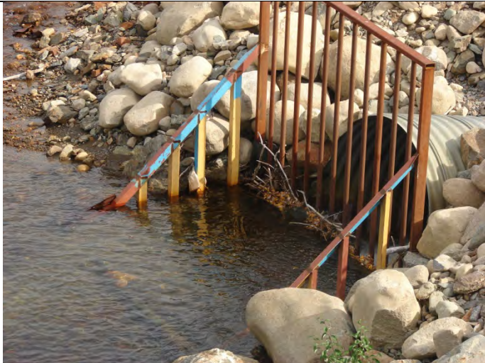
Photograph 13: Looking at the Plunge Pool on a 1,800 mm diameter CSP Culvert inlet, at station 1+1300 – 09-10-2013
