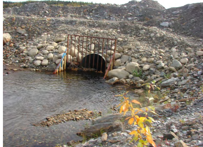
Photograph 14: Looking south at the Plunge Pool on a 1,800 mm diameter CSP Culvert inlet, at station 1+1300 – 09-10-2013
