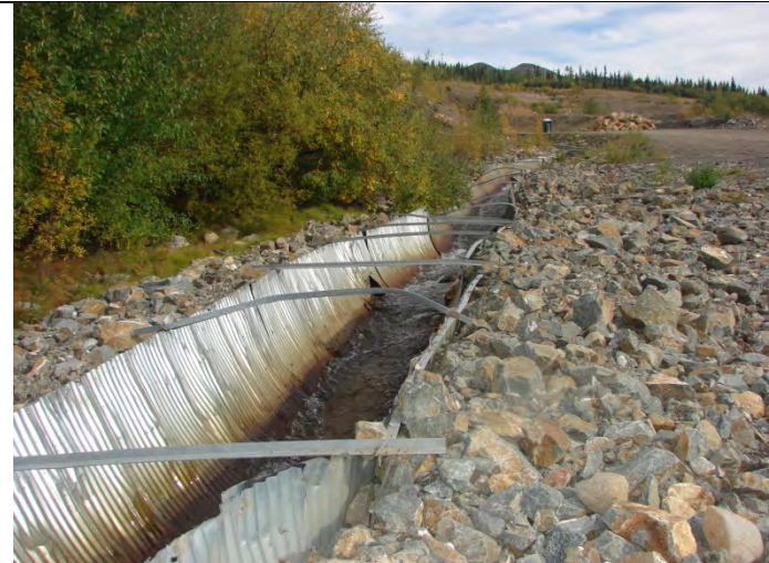
Photograph 10: Looking at half-round 2,400 diameter CSP Culvert, showing instability and failure at some locations – 09-10-2013
