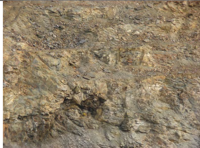
Photograph 38: Looking at Vangorda Pit side walls, showing rock raveling and slumping failures (4) – 09-10-2013
