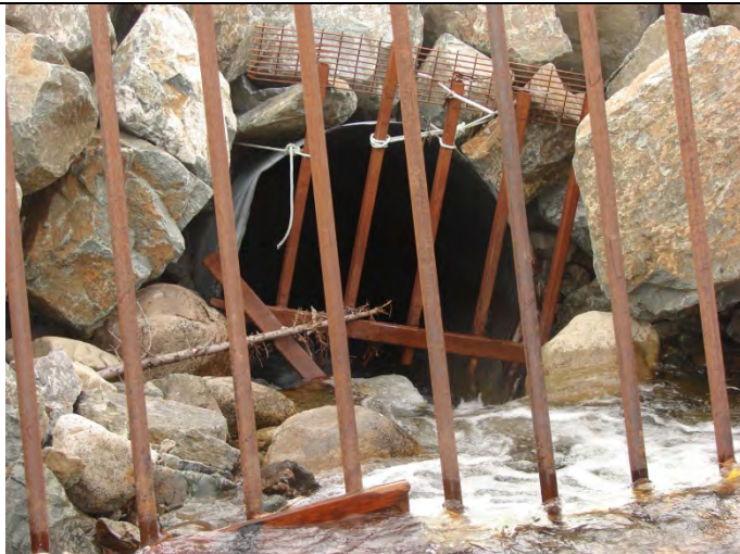
Photograph 31: Looking at the existing 1,500 mm culvert inlet on Vangorda Creek north of access road (1) – 09-10-2013
