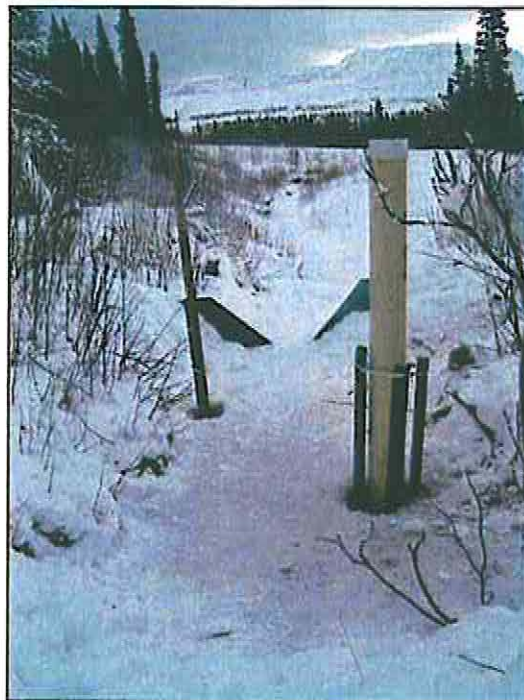
Plate 4 Stilling Well and Staff Gauge Installed Up-Stream of Weir (Looking Downstream)
